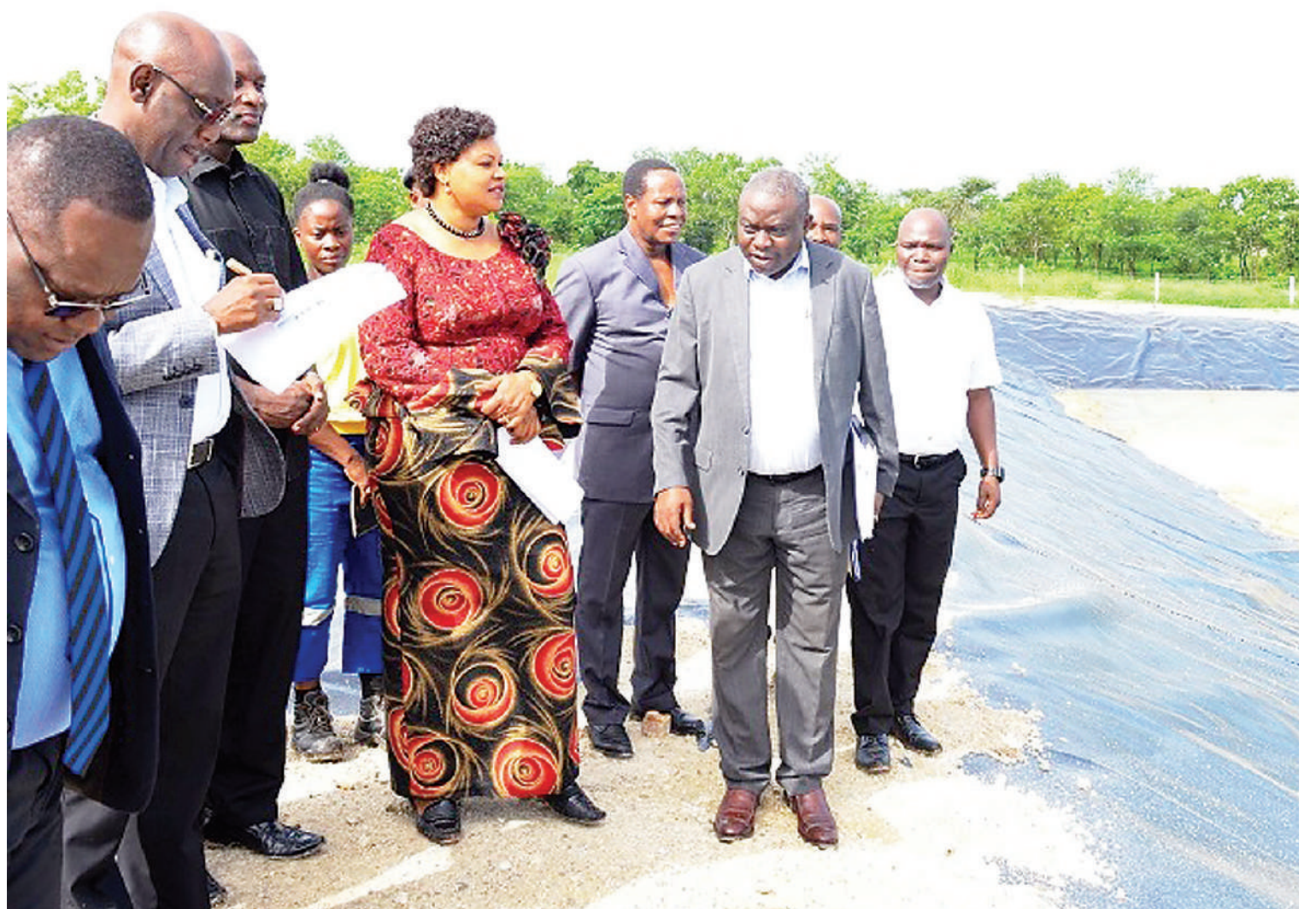
Jenista Mhagama (C), Minister of State in the Prime Minister's Office (Policy, Parliament, Employment, Youth and Persons with Disabilities), pictured on Thursday touring a dam being constructed in the Nguru Hills Ranch in Mvomero District as part of a slaughterhouse project. The dam is meant as a reservoir for treating effluent from the slaughterhouse for subsequent use in irrigation farming. Photo: PMO
