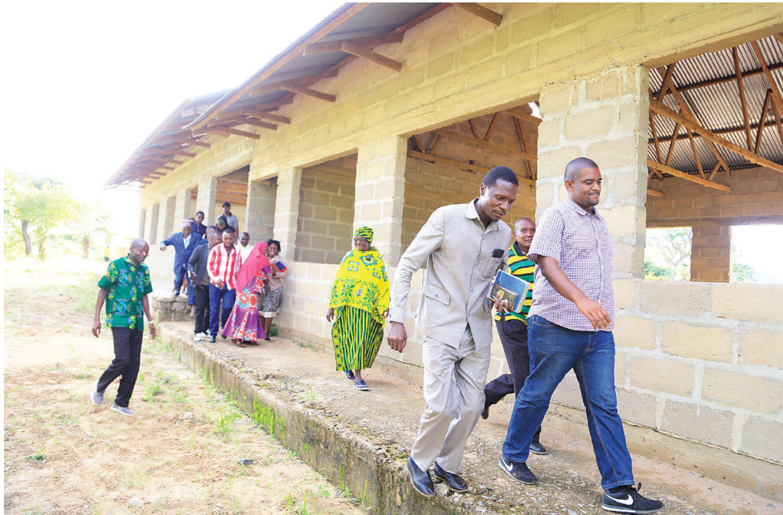
Chamwino legislator Deogratius Ndejemi (R, foreground) has a first-hand account of progress on the construction of classrooms at Itiso Secondary School in Chamwino District on Thursday. Photo: Correspondent Ibrahim Joseph
