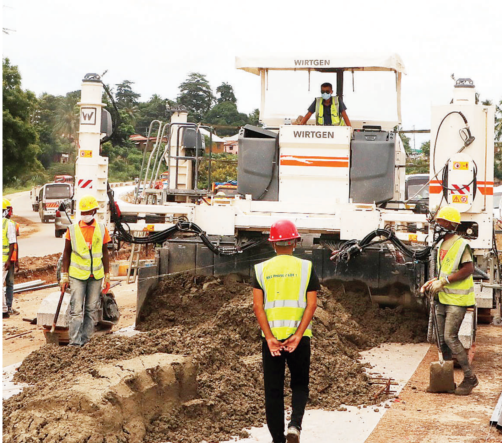
Work on infrastructure for Dar es Salaam's rapid bus project in progress at Kurasini along the Gerezani-Mbagala stretch of Kilwa Road yesterday. Photo: Correspondent Jumanne Juma
