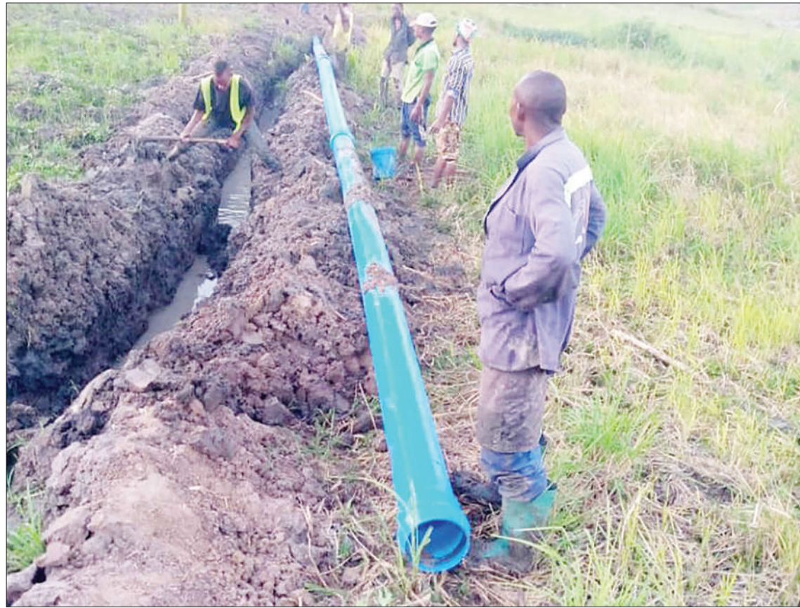
Technicians with Dar es Salaam Water and Sanitation Authority (DAWASA) continue with the implementation of Bangulo B water project by laying down water pipes. The project will save over 2,000 residents of Gongo la Mboto and Pugu in the outskirts of Dar es Salaam. Photo: Correspondent Joseph Mwendapole
