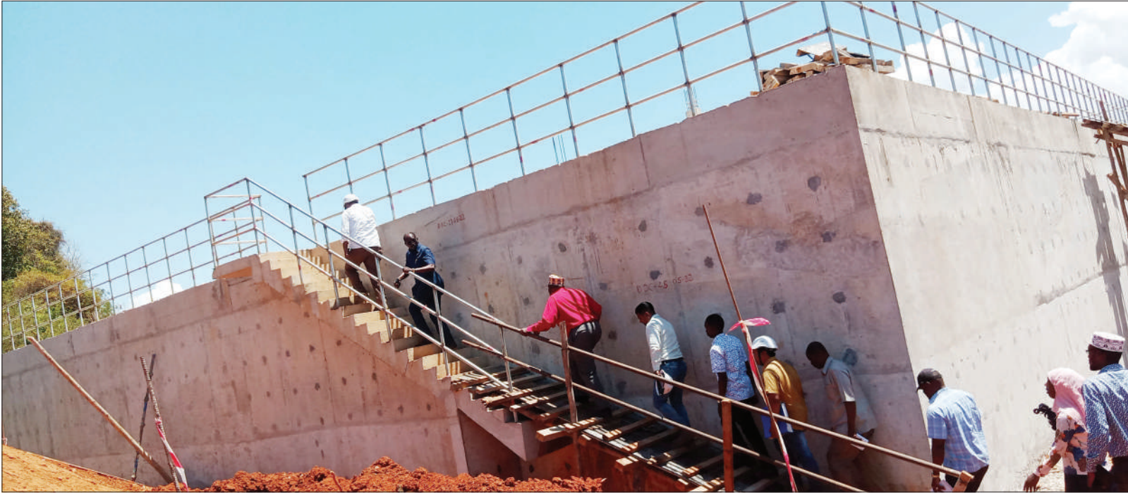
Zanzibar Water, Energy and Minerals permanent secretary, Joseph Kilangi (2nd L), leads officials to inspect a water tank at Dimani constituency in Unguja yesterday. Photo: Rahma Suleiman
