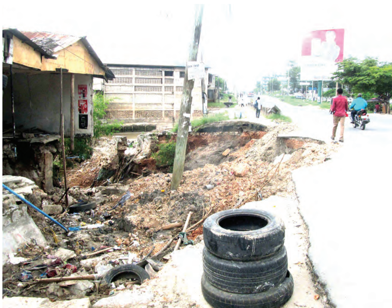
Going, going almost gone. A section of Shekilango road in Sinza suburb on the outskirts of Dar es Salaam after it was washed away by floods recently. Photo: Guardian Correspondent
