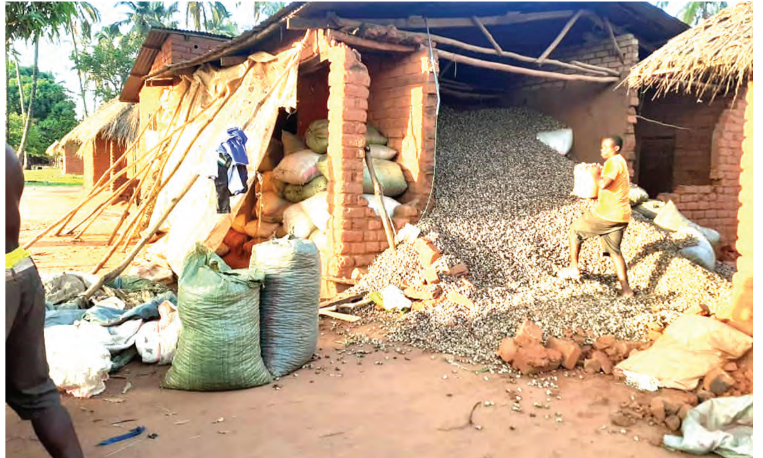
One of 21 go downs belonging to Tunduru district agricultural marketing co-operative societies had been demolished while cashew nut stored in danger of rotting away. Photo: Correspondent Steven Chindiye.
