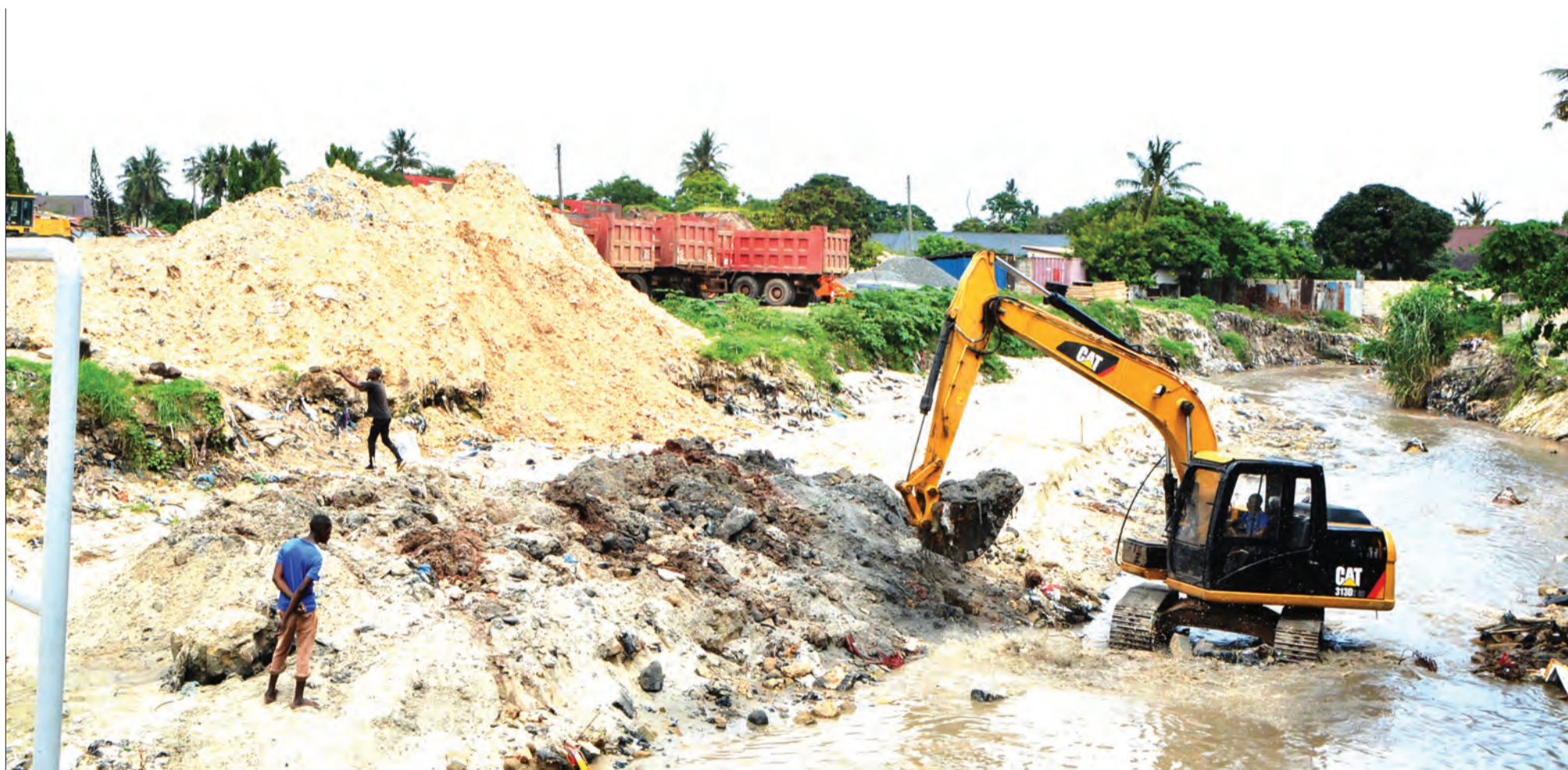
Excavator at work along river Ngo'mbe at Tandale area in the outskirts of Dar es Salaam as captured yesterday. Photo: Correspondent Miraji Msala
