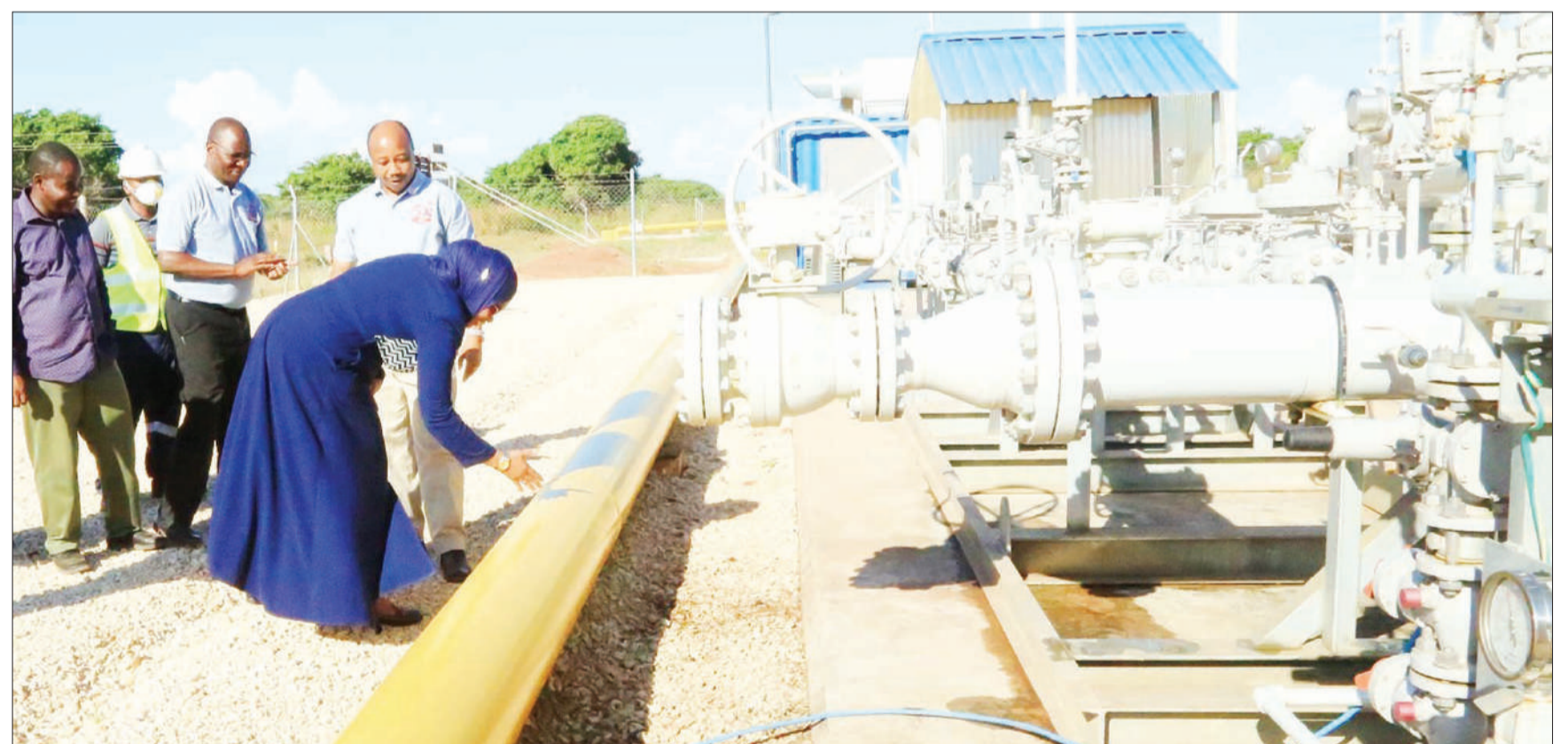
Energy ministry permanent secretary Zena Said touches a pipe used in transporting natural gas while on a just-ended visit to a gas project in Lindi Region. Photo: Correspondent Zuwena Msuya
