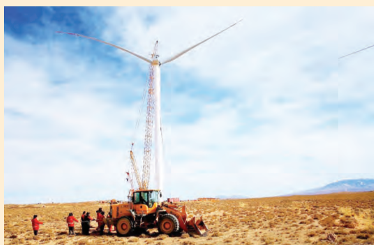
A wind turbine is being erected in a 30-kW wind farm in Ganzhou district, Zhangye, northwest China's Gansu province, Feb. 10, 2023. (Photo by Yang Yongwei/People's Daily Online)
