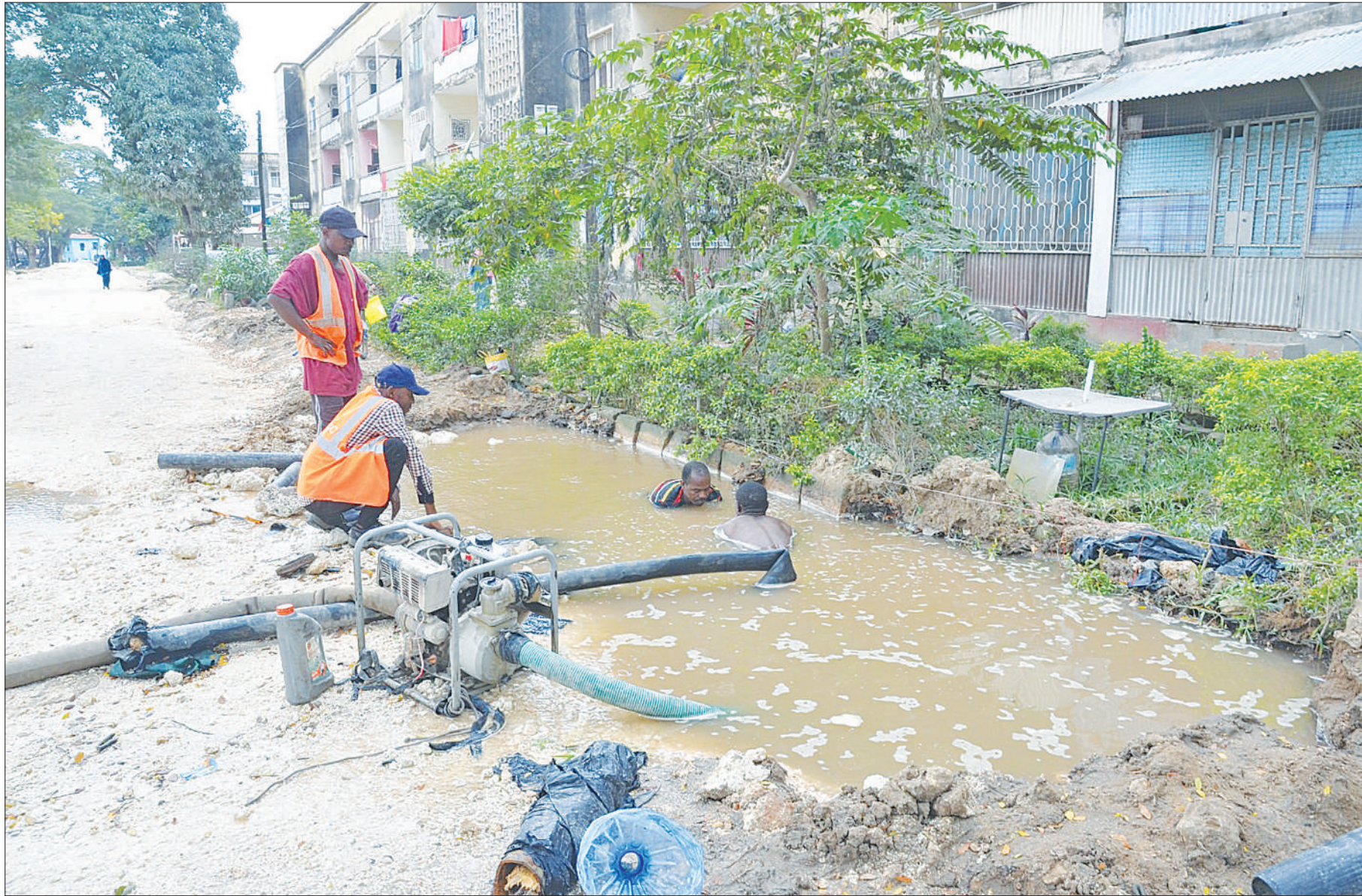
Contractors rehabilitating the road linking Zanzibar's Mnazi Mmoja suburb to the former Zanzibar House of Representatives complex at Kikwajuni are forced to repair a clean and safe water pipe first yesterday before proceeding with their work. Photo: Rahma Suleiman
