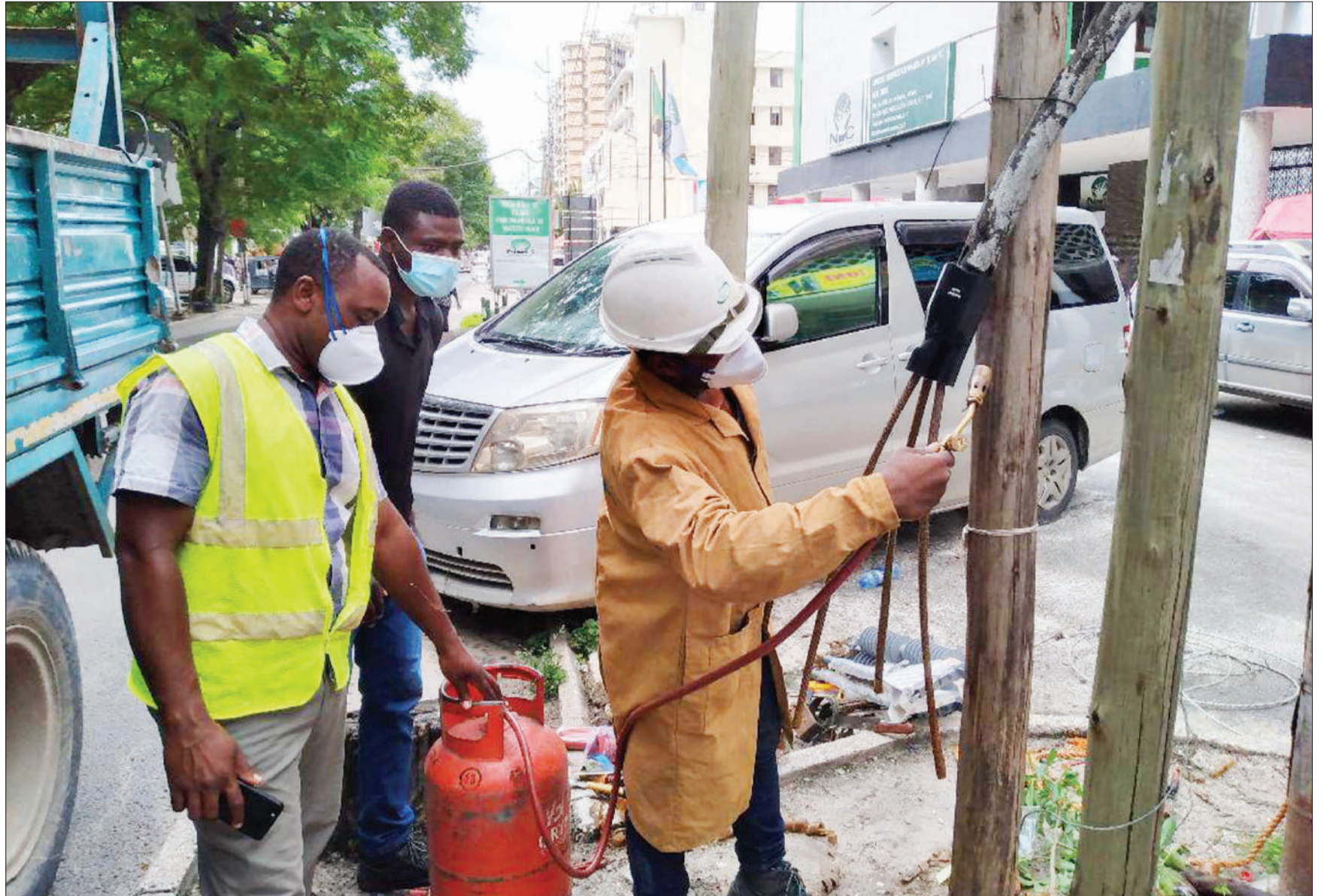
Tanzania Electric Supply Company (TanESCO) technicians move to repair defective cables along Samora Avenue in Dar es Salaam yesterday. Photo: Correspondent Joseph Mwendapole
