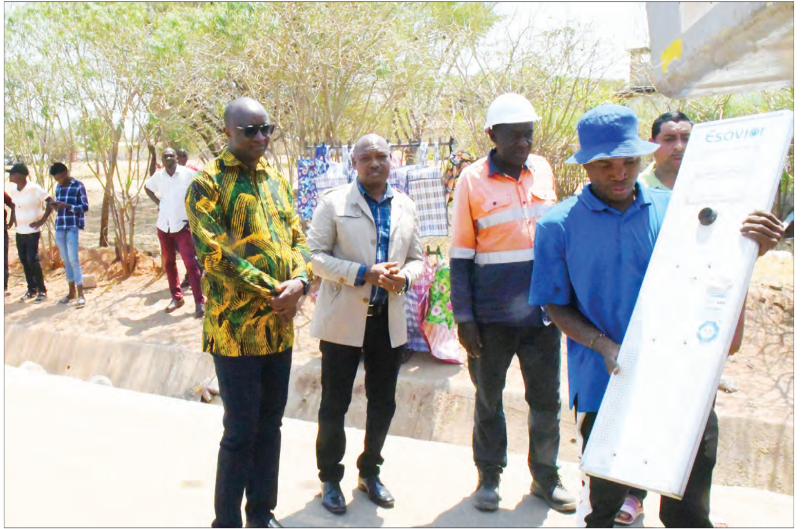
One of the technicians installing solar-powered road traffic lights in Shinyanga municipality briefs Shinyanga regional commissioner Dr Philemon Sengati (L, foreground) yesterday on what the work involves. Photo: Vicent Tiganya
