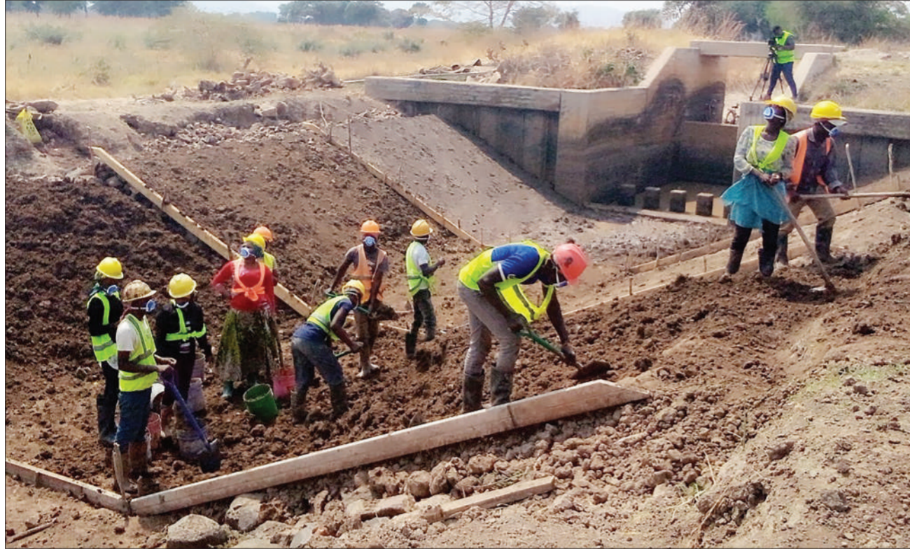
Construction of water canals and drainage systems, which is in implementation of the Madibira irrigation scheme in Mbarali District, has reached half-way stage. The drive is part of the World Bank-funded Resilient Natural Resources for Growth (REGROW) project, whose thrust is on transform the tourism sector in Tanzania's southern circuit. Photo: Felister Peter
