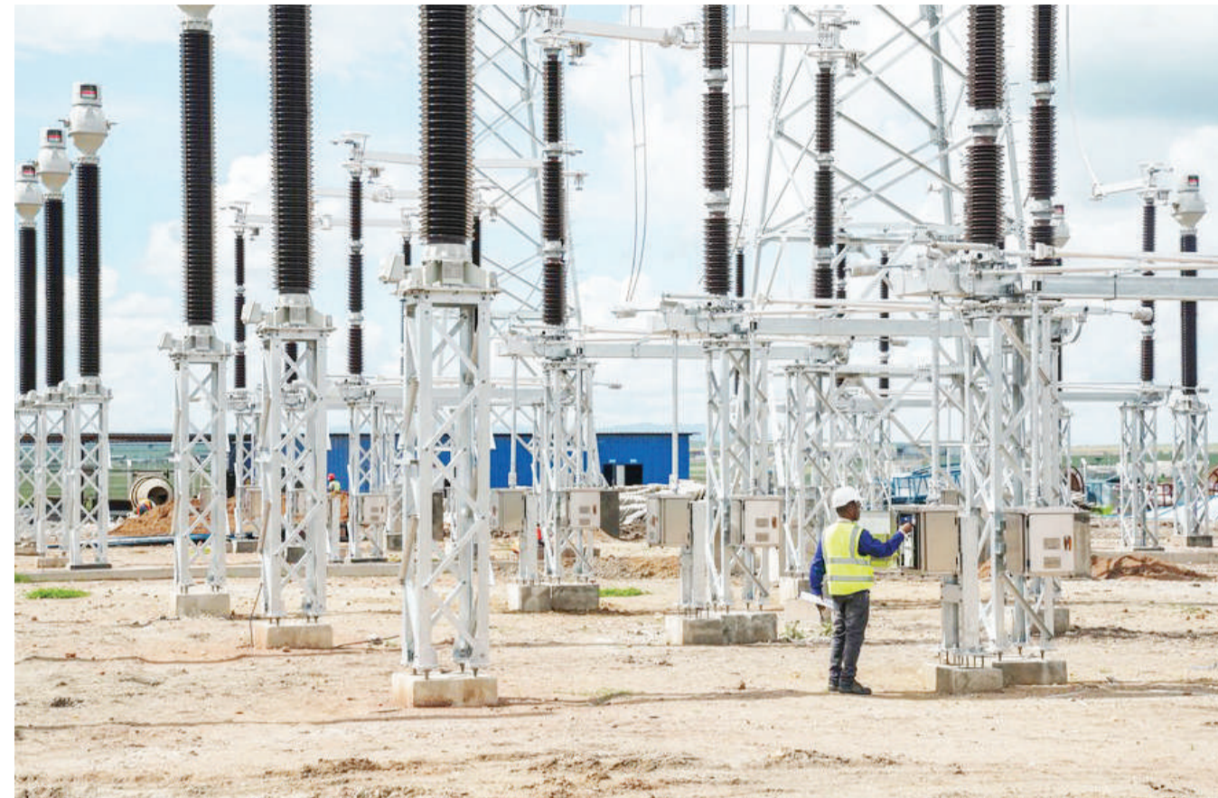
David Maina Kamore patrols at the construction site of the Konza transformer substation in Machakos County, Kenya.
