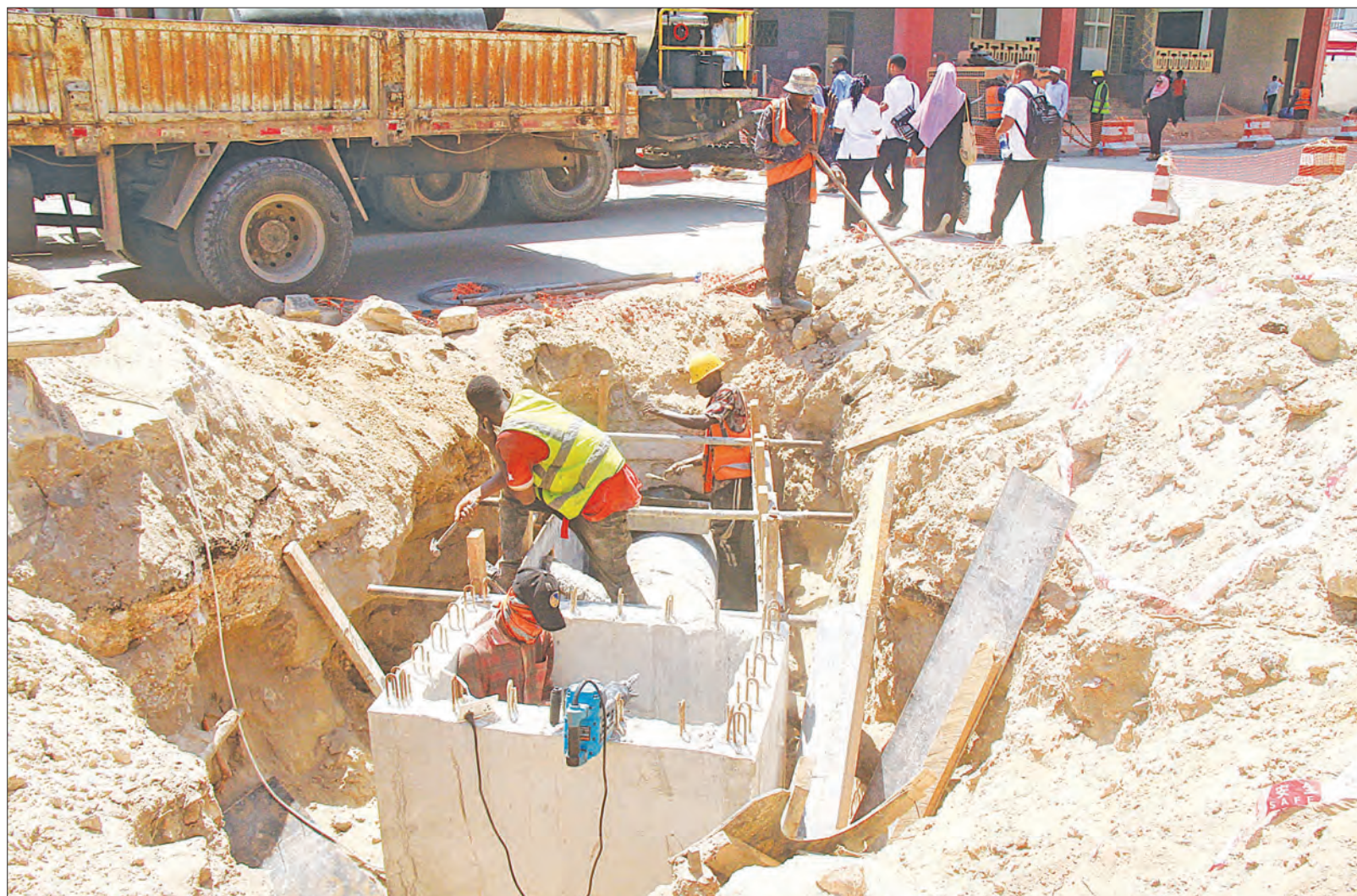
Work on a floodwater drainage chamber constituting part of the ongoing implementation of the Bus Rapid Transit (BRT) road infrastructure project in progress at a spot in downtown Dar es Salaam yesterday. Photo: Correspondent Jumanne Juma
