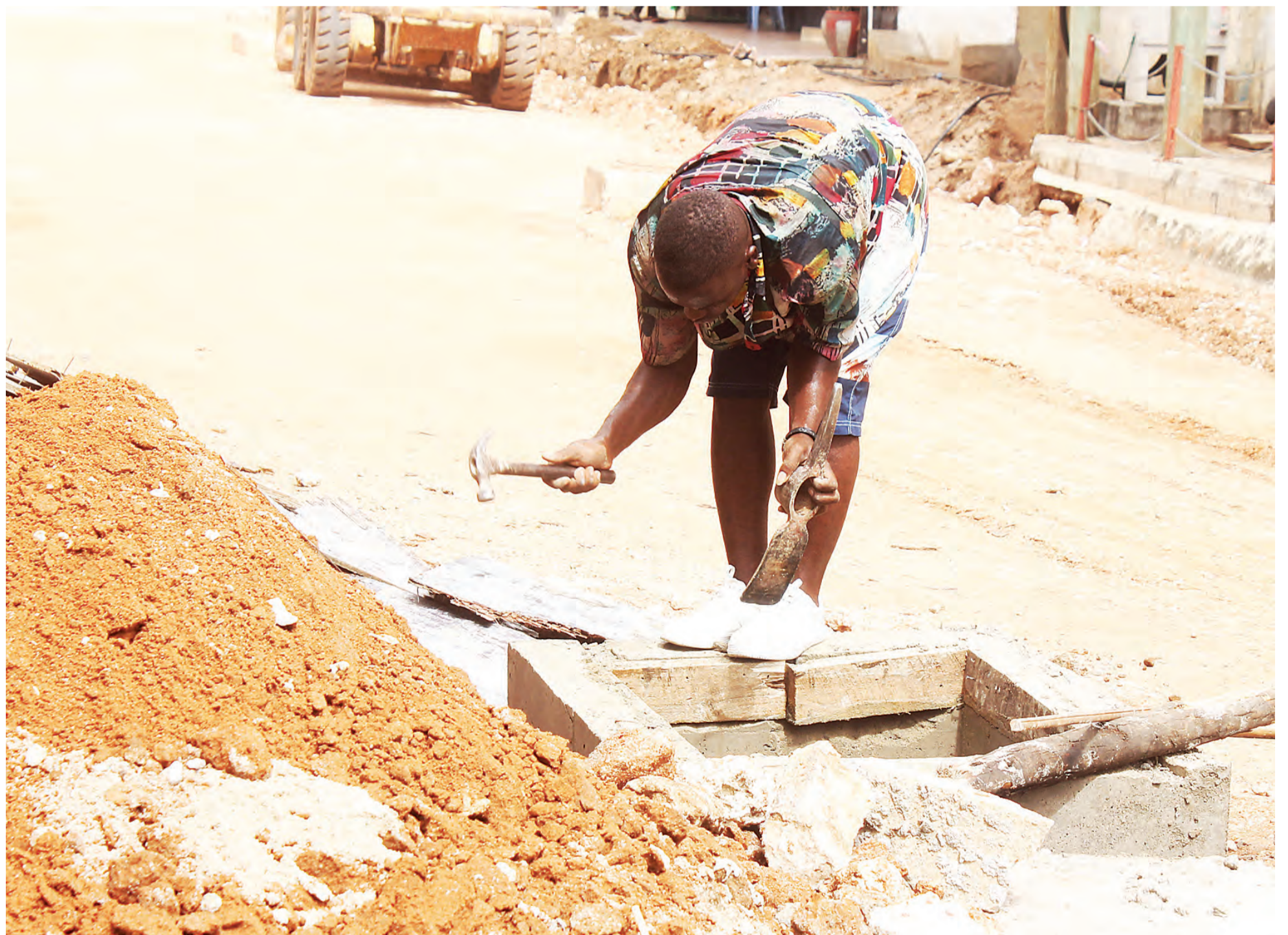
A Tanzania Rural and Urban Roads Agency technician works on a drainage system along a street in Dar es Salaam's sprawling Kariakoo market zone yesterday. Photo: Correspondent Jumanne Juma
