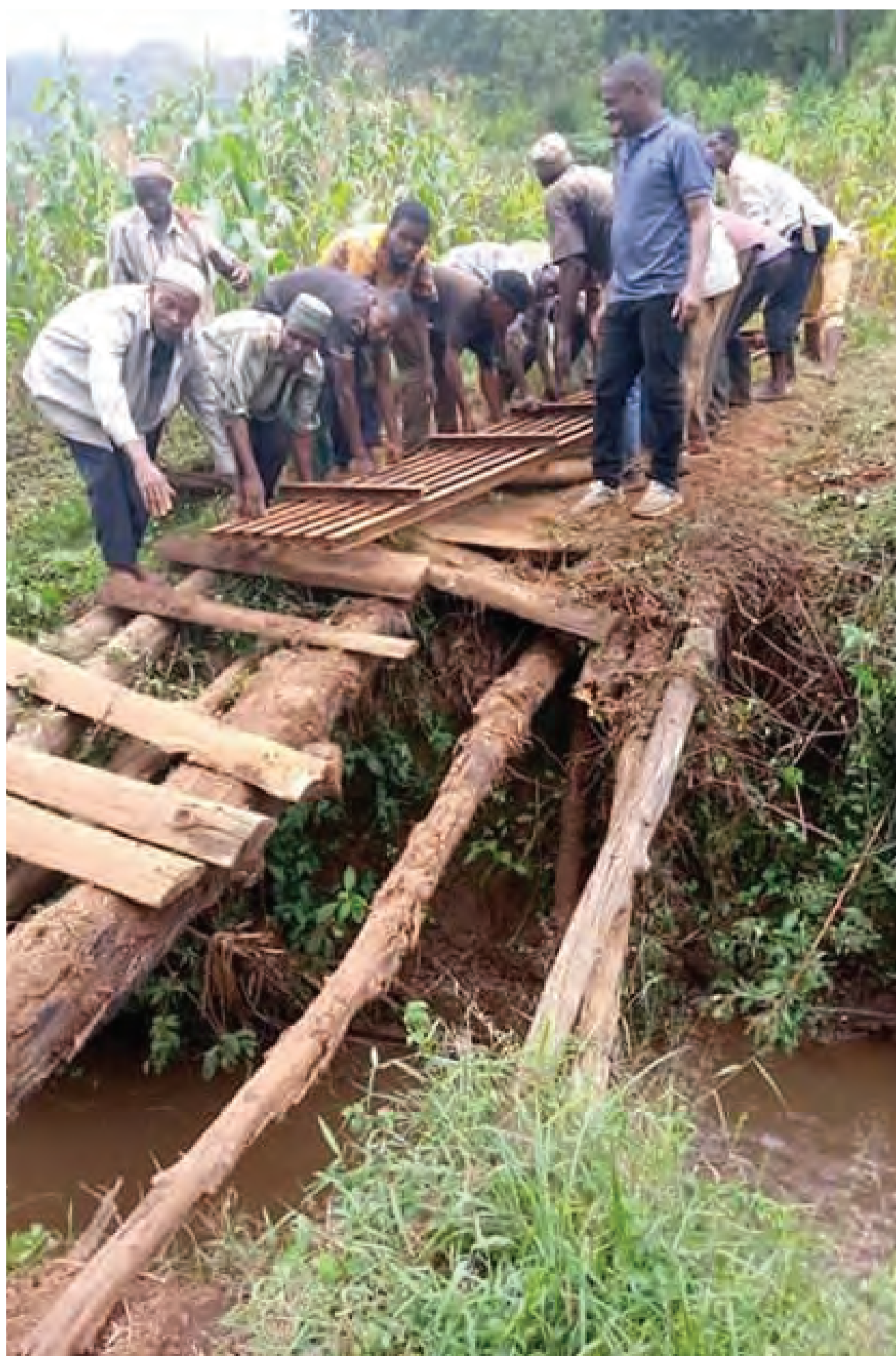
Residents of Vuga ward in Lushoto District pictured yesterday building a temporary bridge in the place of the one formerly there, which has been swept away by floodwaters. Photo: Correspondent Boniface Gideon
