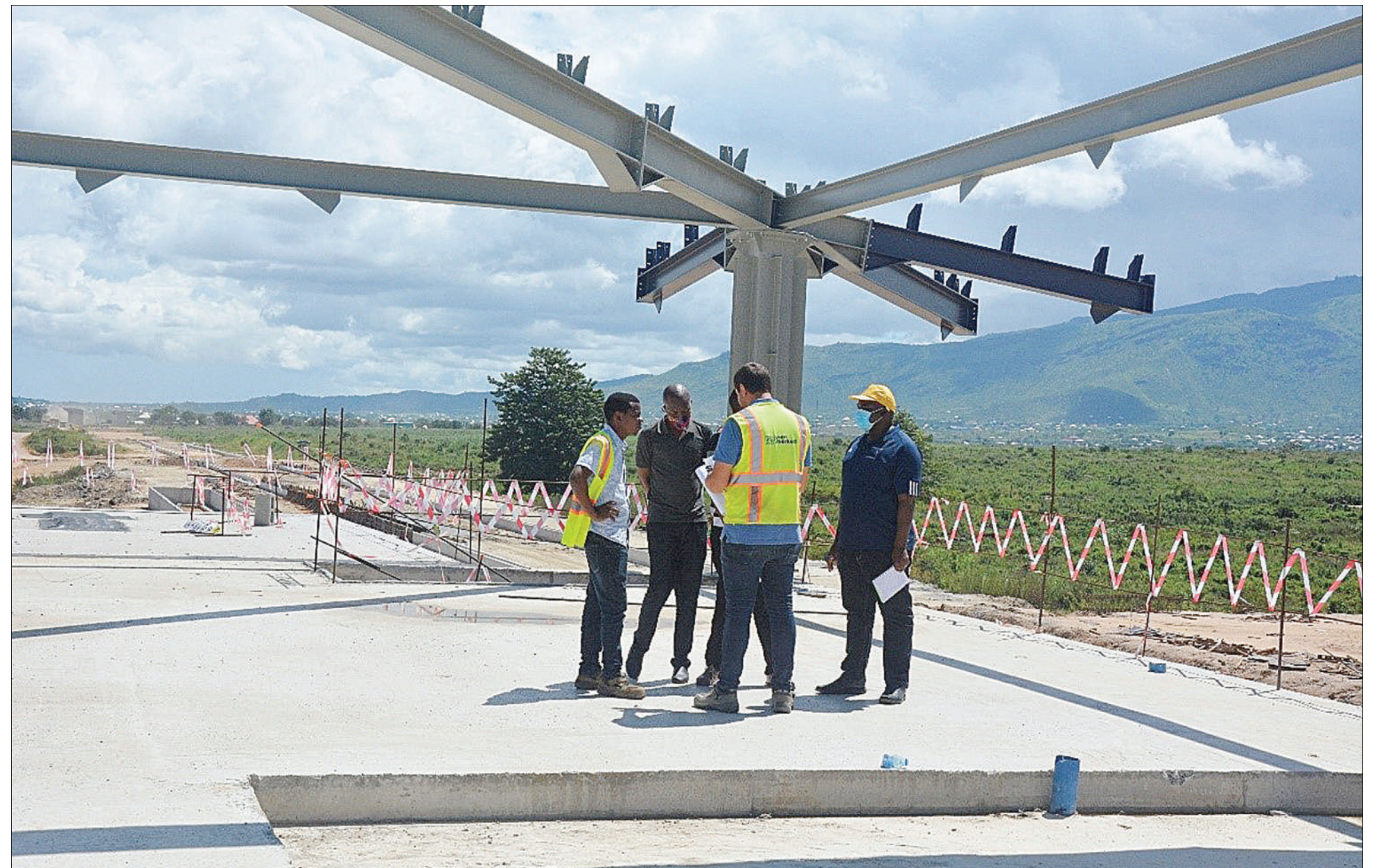
Lands, Housing and Human Settlements Developments ministry planning officers have a word with Standard Gauge Railway project engineers in Dar es Salaam yesterday on matters related to cooperating with the Tanzania Railway Corporation in ensuring work at major SGR major stations does not lead to the growth of unplanned urban settlements. Photo: Guardian Correspondent
