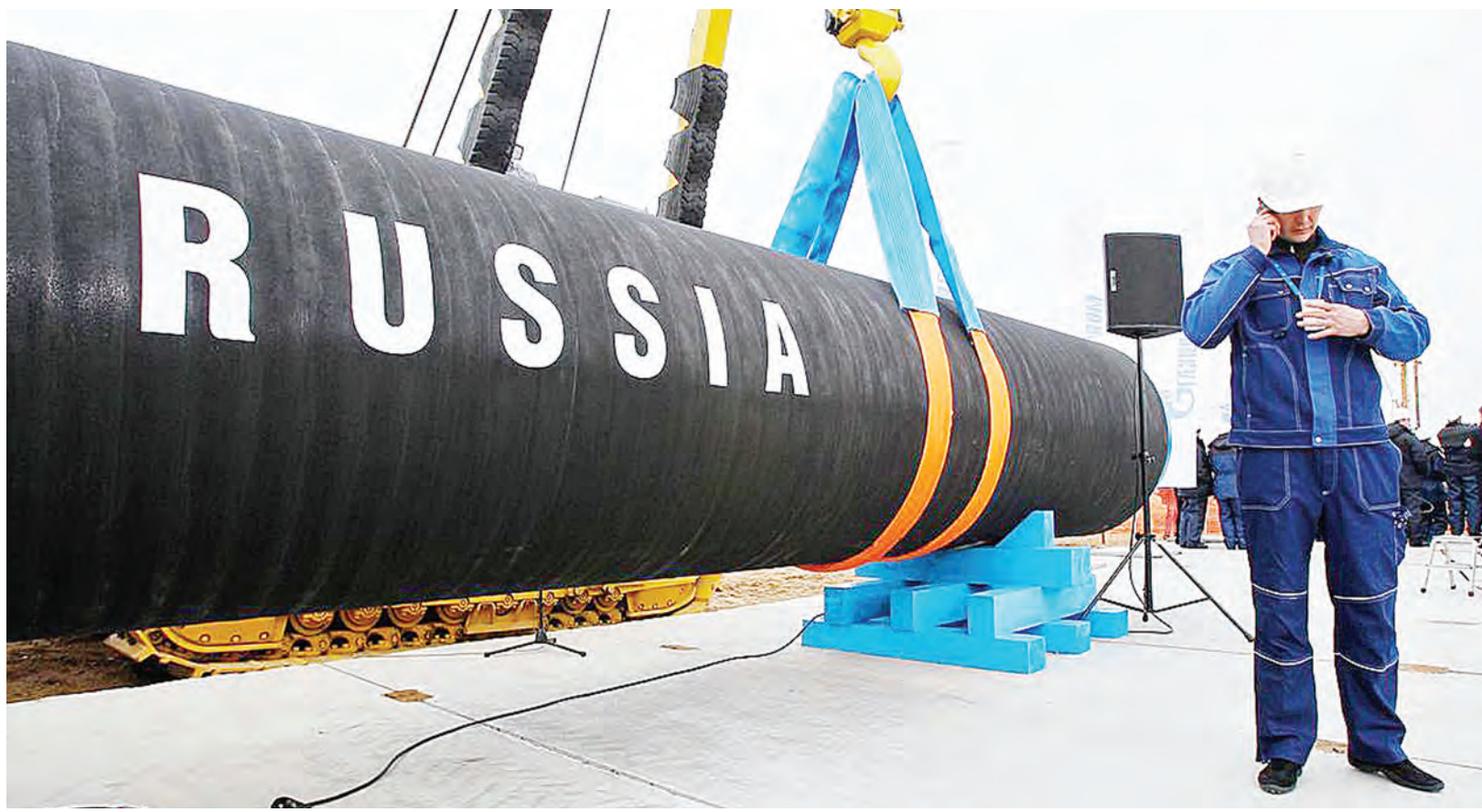
A Russian construction worker on his phone at the laying of a section of the Nord Stream 2 pipeline between Russia and Germany. Nord Stream 2 is owned by Gazprom, with investment from several European companies including Shell, Engie, OMV and Wintershall Dea.
