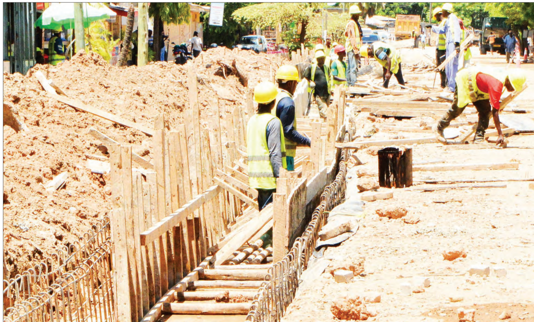
Employees at work during the ongoing expansion of Shekilango road at Sinza Mori suburb in Dar es Salaam yesterday. Photo: Correspondent Miraji Msala
