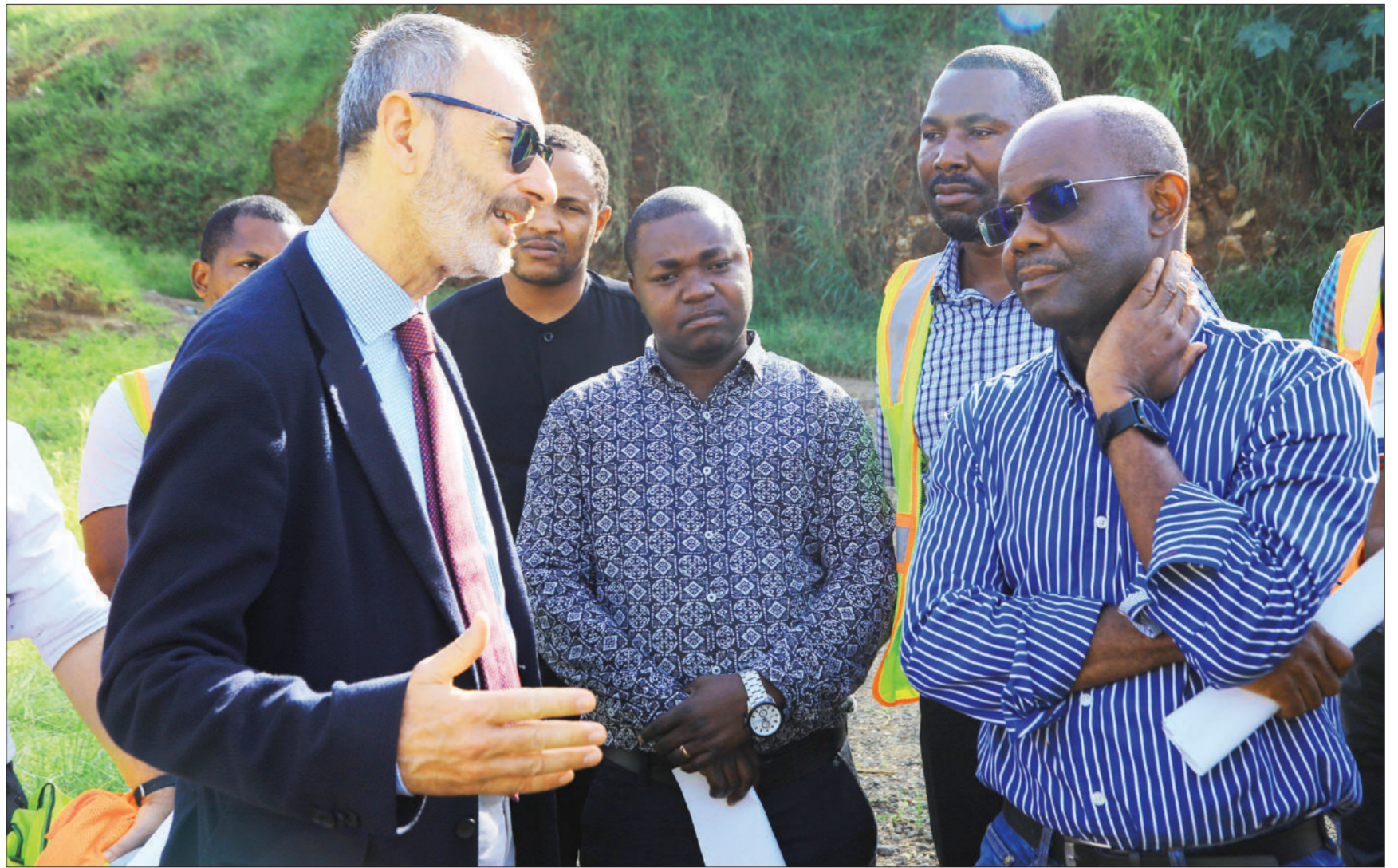
The European Union's Ambassador to Tanzania, Manfredo Fanti (L), has a word with Works and Transport minister Prof Makame Mbarawa (R) during an inspection tour of the ongoing construction of the 66.9-km Kidatu-Ikafara road in Morogoro Region at the weekend. Photo: Guardian Correspondent
