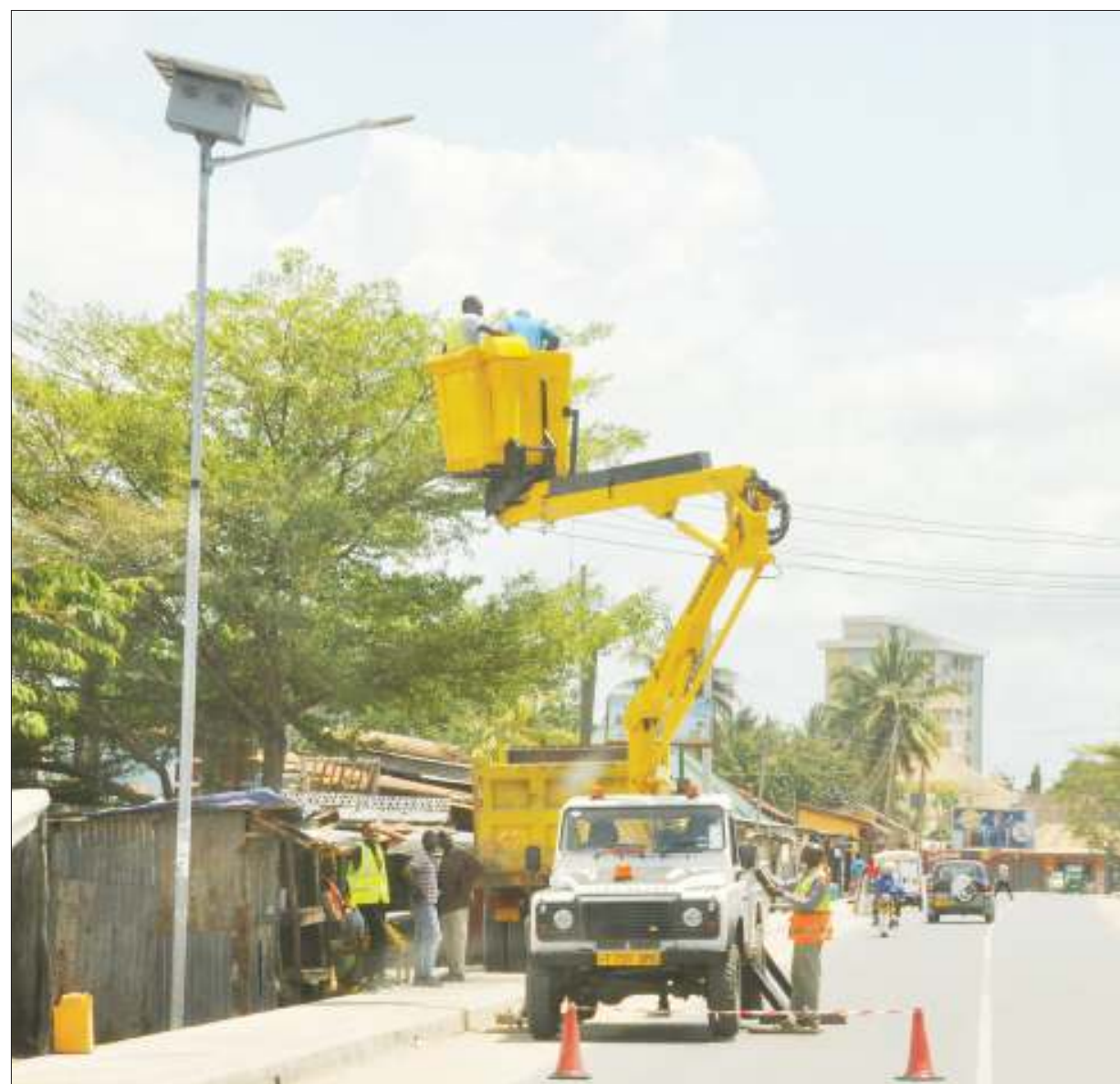
Technicians install a solar energy light pole at Temeke kwa Sokota in Dar es Salaam at the weekend. Photo: John Badi
