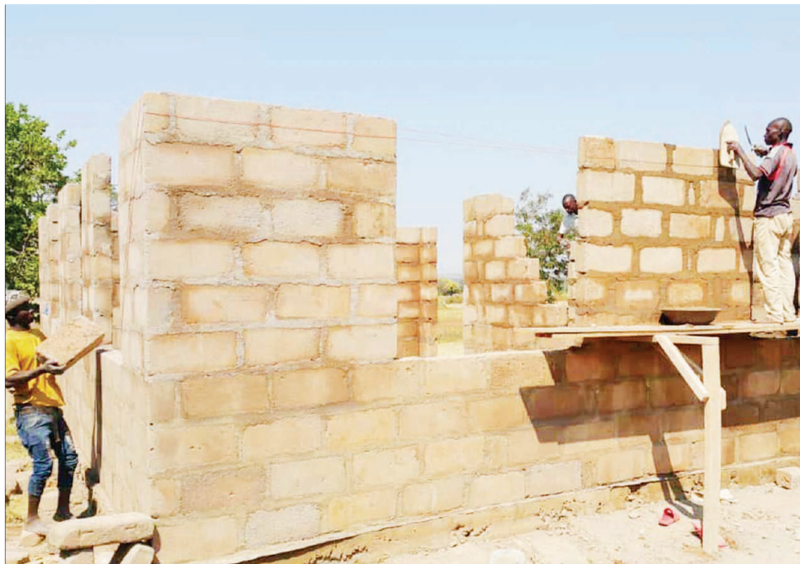
Construction of a classroom building meant for students with special needs in progress at Nyambono B Primary School in Musoma Rural constituency earlier this week. Photo: Guardian Correspondent
