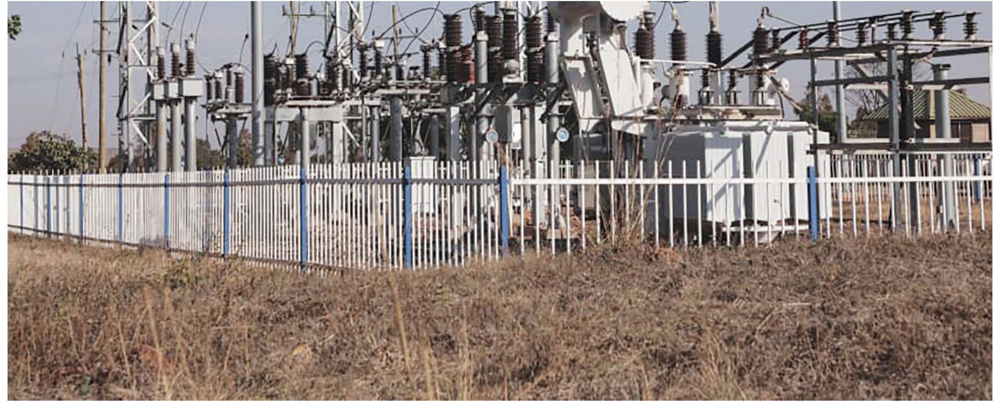
The 33/11 KV Kibongo Grid electricity receiving and Cooling Station at Kibondo.
