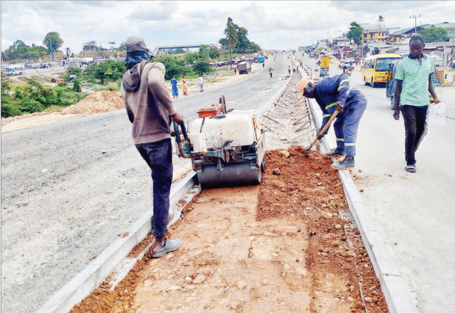
Work on the newly expanded road leading to the Magufuli main bus stand at Mbezi Luis in Dar es Salaam's Ubungu municipality is nearing completion, as captured yesterday. Photo: Correspondent Sabato Kasika
