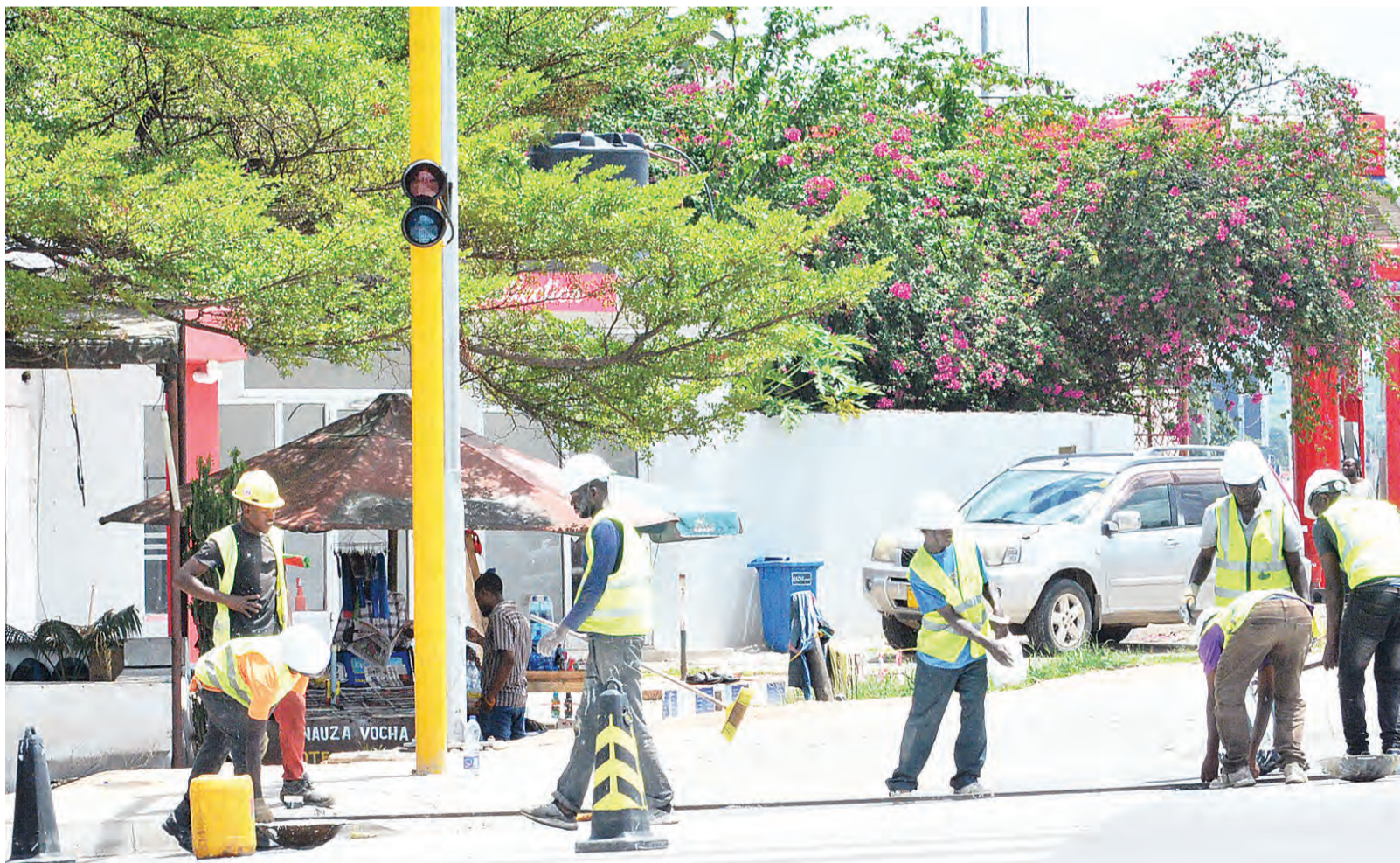
Construction workers painting zebra crossing sign on Shekilango road within Kinondoni municipality in Dar es Salam earlier this week. Photo: Correspondent Miraji Msala
