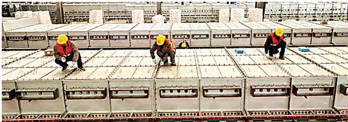
Construction workers install equipment at a construction site of a lithium battery project on April 6, 2023 in Renshou County, Meishan City, Sichuan Province of China. Photo: Vcg/Visual China Group/Getty Images
