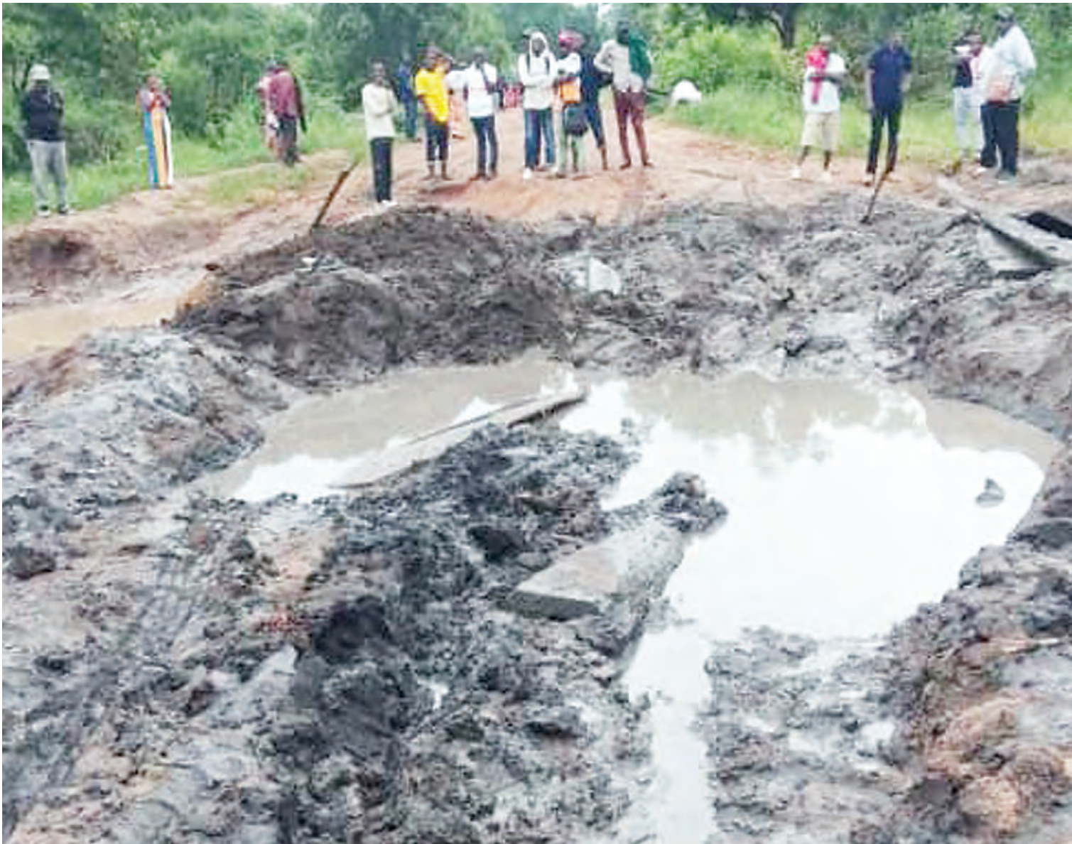
Passers-by have a curious view of gaping potholes along the Mlowoka stretch of the Nangurukuru-Liwale road in Lindi Region earlier this week, with the damage blamed on the ongoing rains. Photo: Guardian Correspondent
