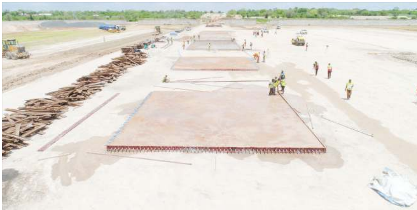
Work has begun in earnest on what is meant to develop into Kwala Dry Port in Kibaha District, as captured yesterday. The facility will have capacity to receive and store 3,000 containers at a go, thus substantially easing congestion at Dar es Salaam Port and road traffic jams in the city. Photo: Correspondent Mary Geoffrey
