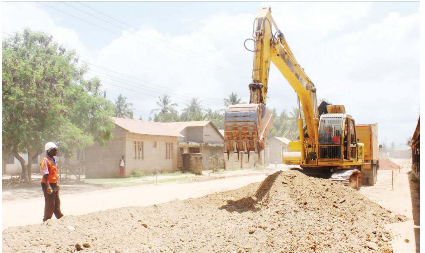
Construction of a road to link Dar es Salaam's Kitunda and Kivule suburbs in progress yesterday. Photo: Correspondent Jumanne Juma
