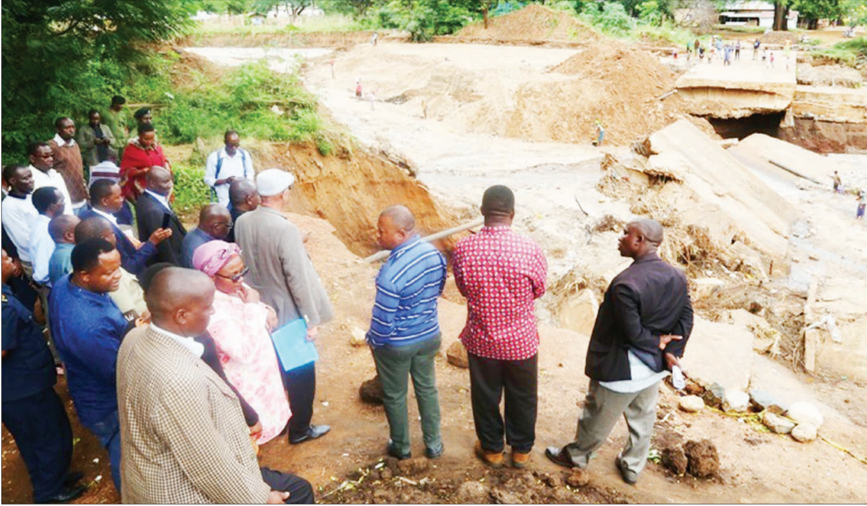
A delegation led by Mussa Hassan Zungu (in cap), Minister of State in the Vice President's Office (Union and the Environment), has a first-hand account yesterday of the damage that ongoing rains in Mpwapwa District have wreaked on strategic Shaaban Robert Bridge. Photo: Guardian Correspondent
