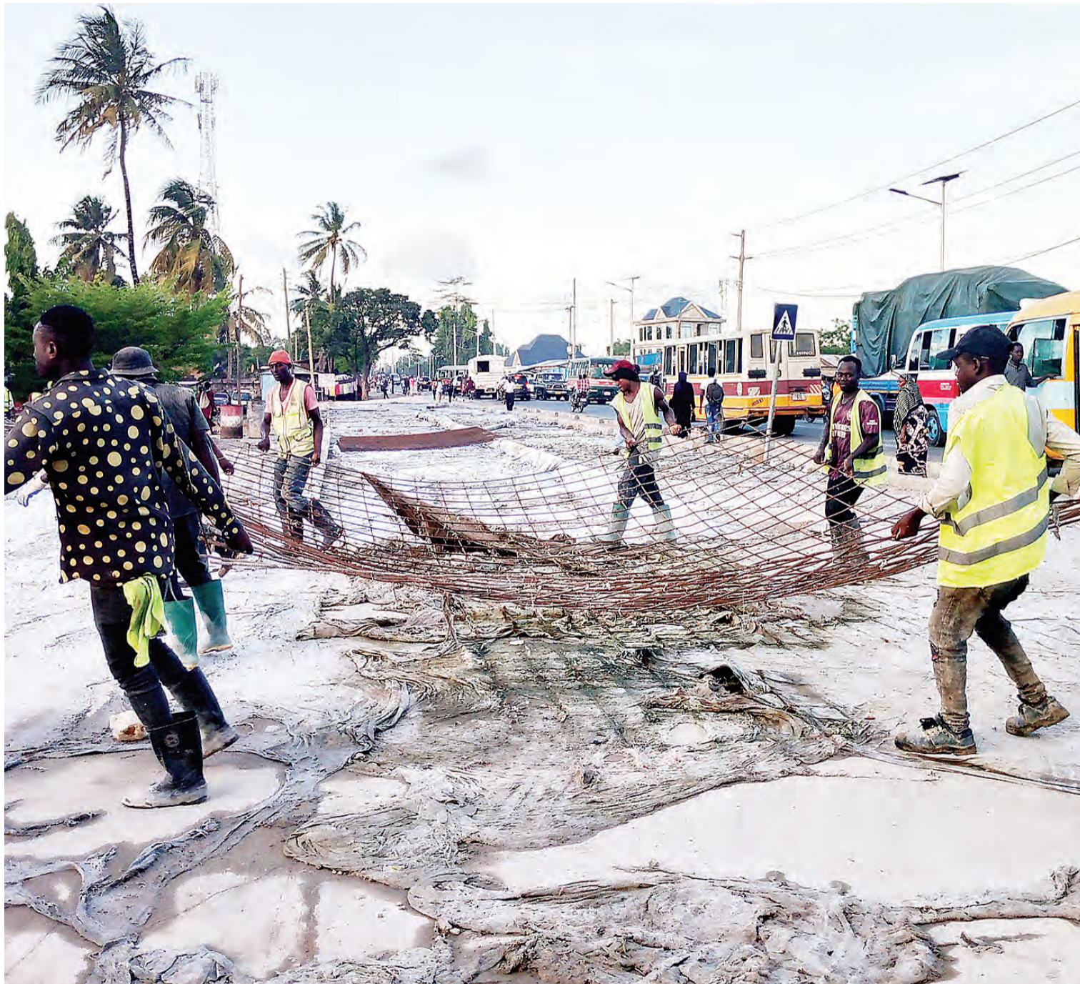
Work has begun on what is meant to grow into a commuter bus stand at Mabibo Mwisho in Dar es Salaam, as found yesterday. Photo: Correspondent Sabato Kasika
