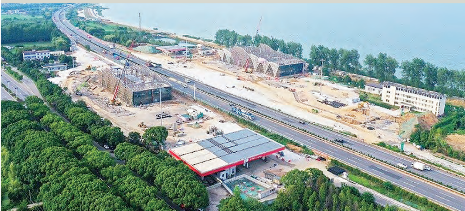
A rest area along the G25 Changchun-Shenzhen Expressway is being constructed in Changxing county, Huzhou, east China's Zhejiang province, June 2022. (People's Daily Online/Chen Haiwei)
