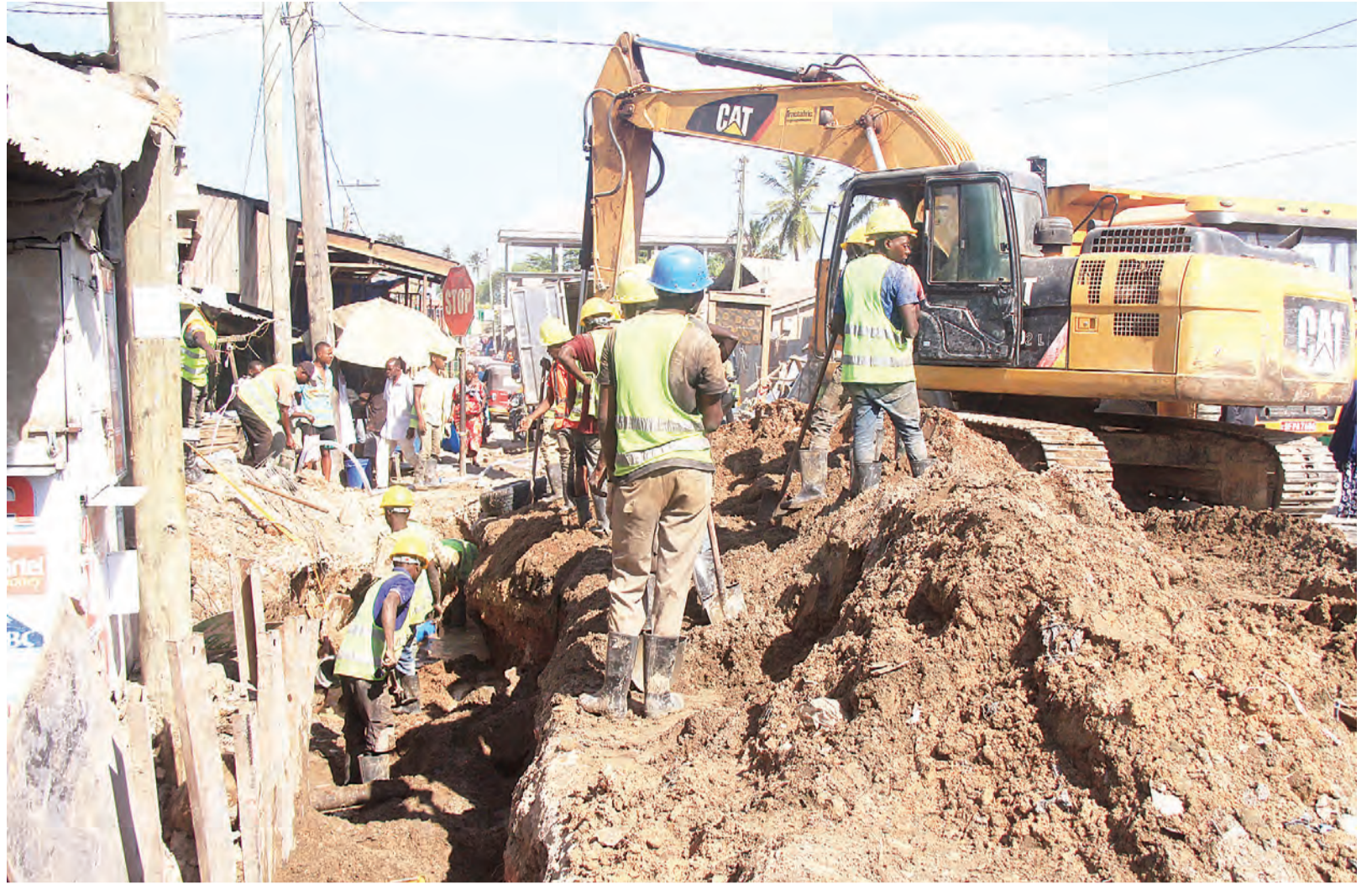
Preparations for the implementation of a water connection, supply and distribution project well in progress in Dar es Salaam's Kitunda suburb yesterday. Photo: Correspondent Jumanne Juma
