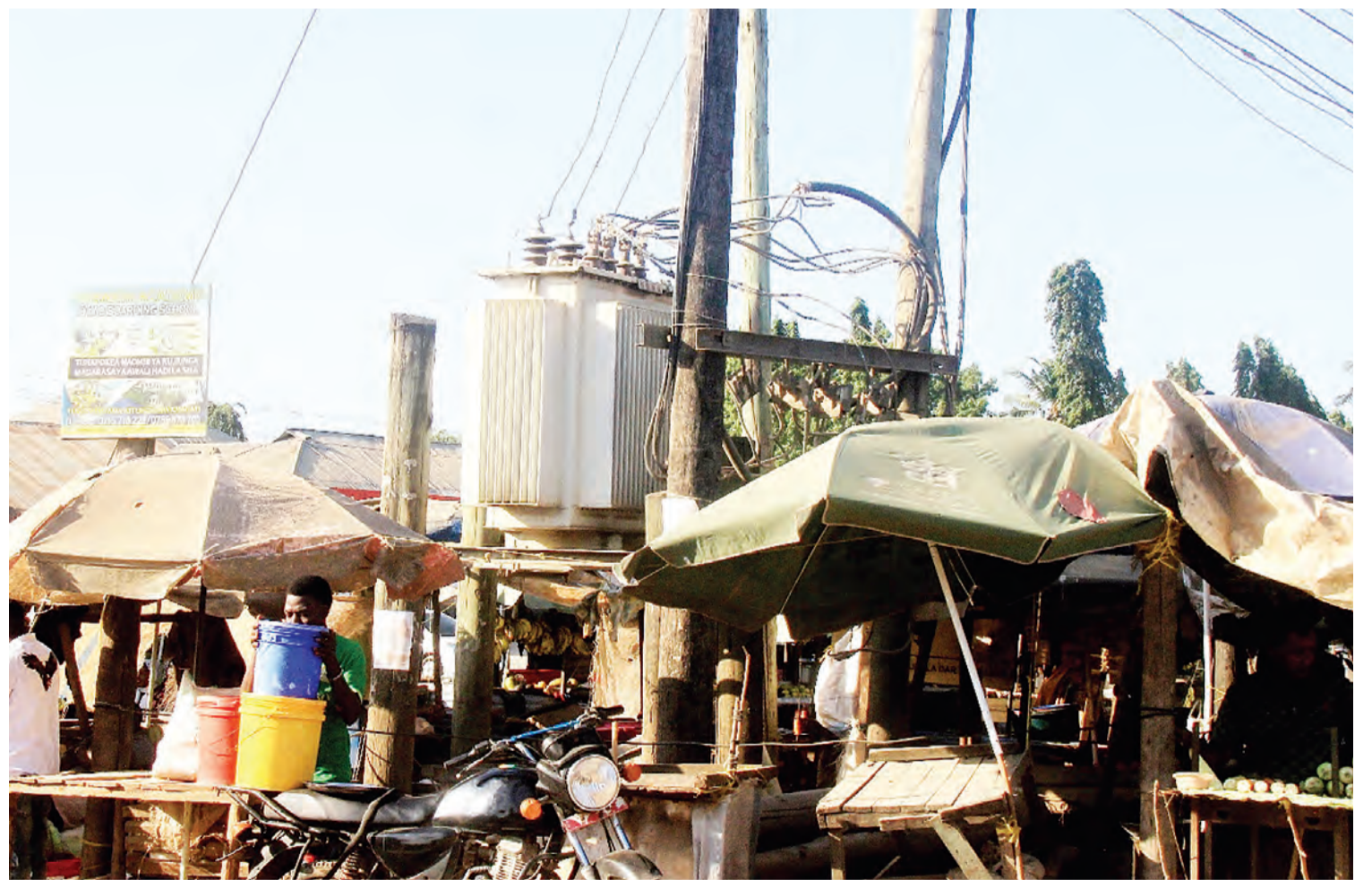
SERIOUS DANGER LOOMS: Small traders pictured yesterday conducting various activities right under - or next to - high-tension power cables and a high-voltage transformer at a makeshift open market in Dar es Salaam's Kitunda suburb. Photo: Correspondent Jumanne Juma
