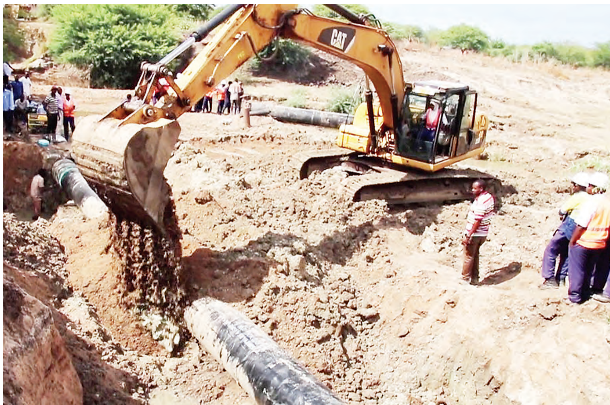
Laying of a new water pipe well in progress in Shinyanga municipality on Thursday under the supervision of the Shinyanga Urban Water Supply and Sanitation Authority. Photo: Correspondent Marco Maduhu
