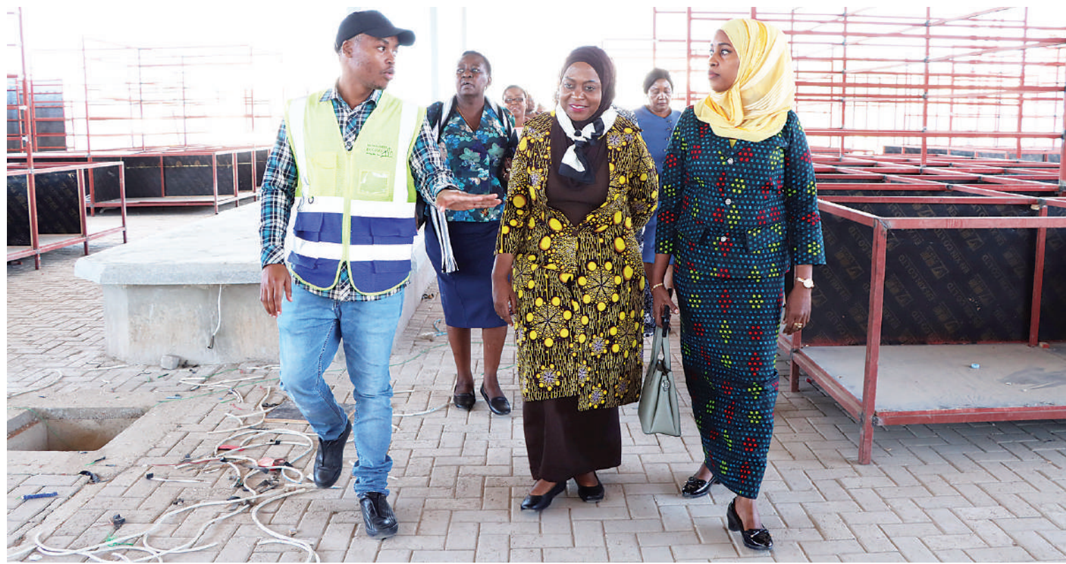
Tanzania Revenue Authority (TRA)'s tax compliance ambassadors Subira Mgalu (2nd-R) with Zulfa Mmaka (R) are shown the various infrastructure of the traders' central market which is under construction in Dodoma during their working visit to show the public how the taxes paid are used in the country. Photo courtesy of TRA
