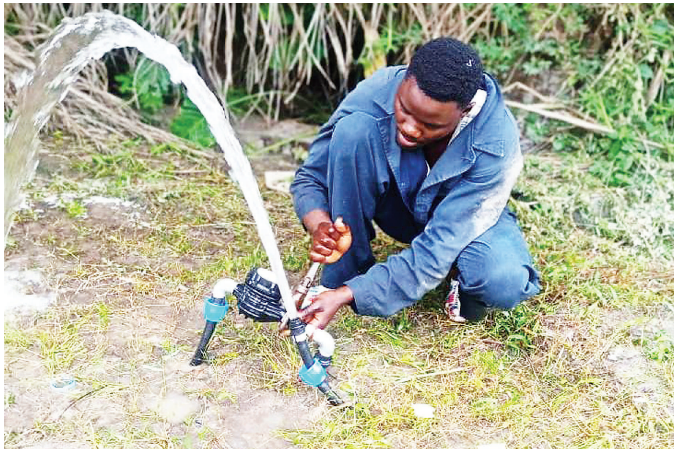
A Dar es Salaam Water Supply and Sanitation Authority (Dawasa) technician who gave his name as Christopher Ernest repairs a water pipe at Kimara Butchery in Ubungo municipality yesterday to ensure reliable supply of potable water to users. Photo: Correspondent Joseph Mwendapole
