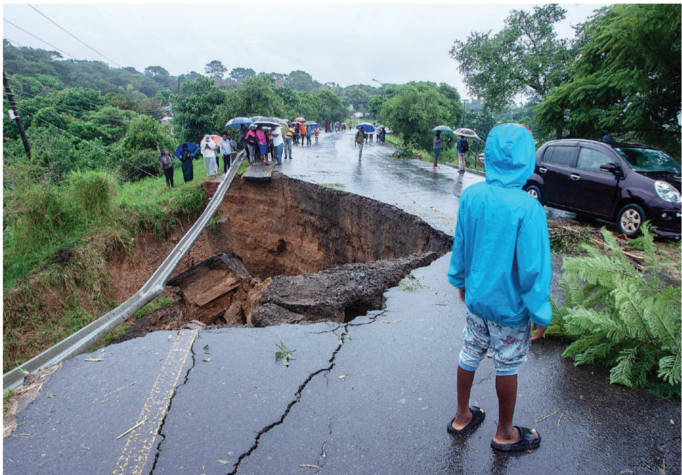
Tropical cyclone Freddy caused severe damage to the coastal communities of Mozambique and Malawi early this year, including destruction of homes, buildings and infrastructure.
