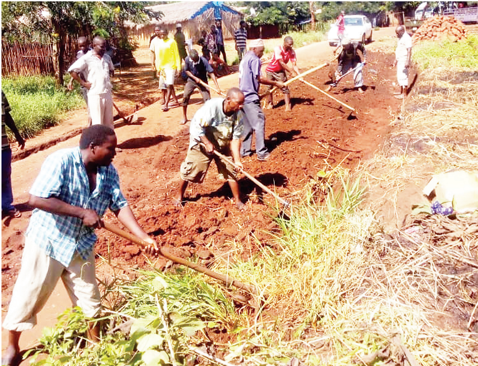
Residents of Kibutuka in Liwale District pictured yesterday repairing a road in the village damaged by rain. Photo: Guardian Correspondent
