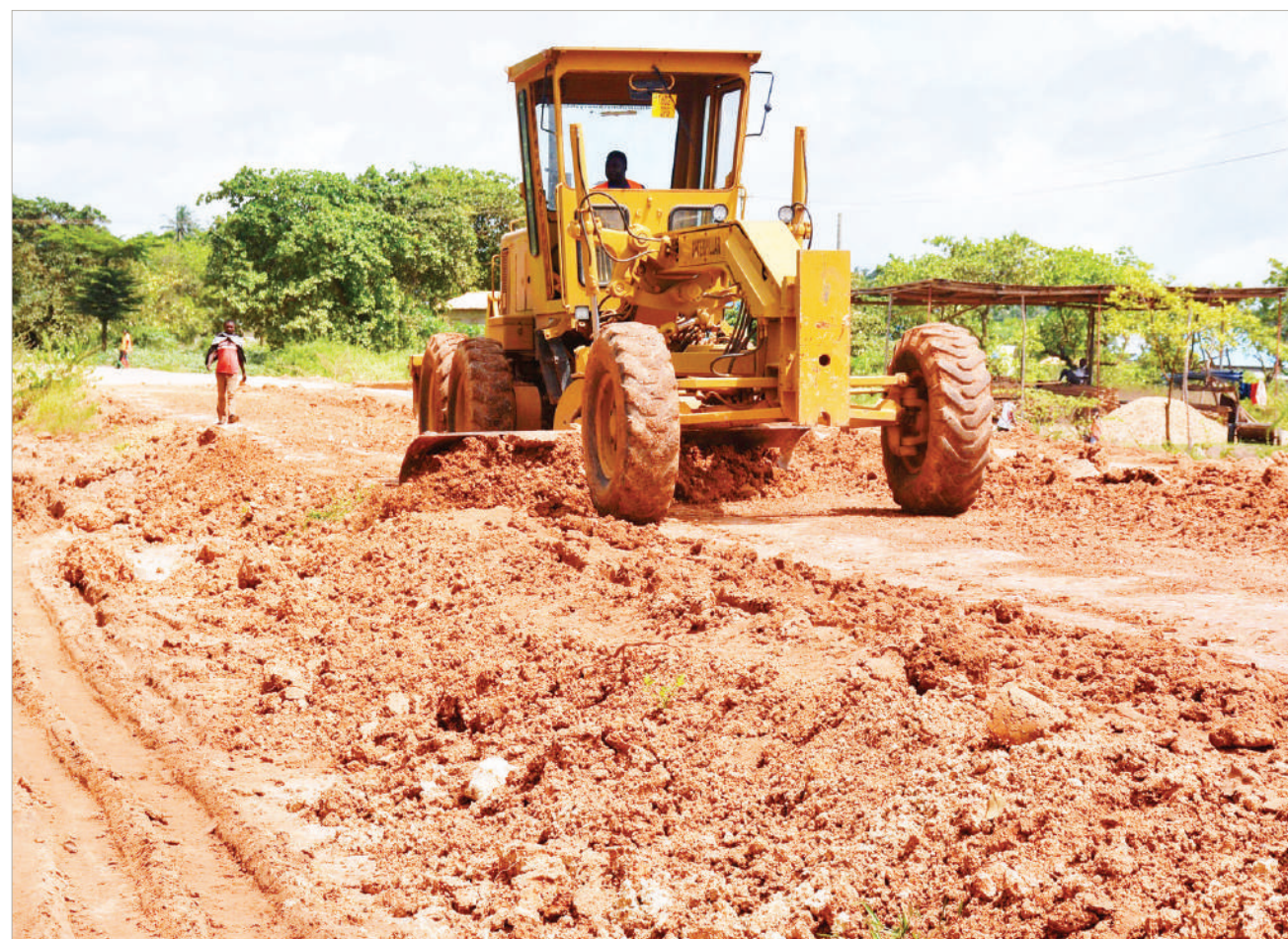
Kitonga section of Chanika road in suburban Dar es Salaam undergoes rehabilitation, as captured yesterday. Photo: Correspondent Jumanne Juma
