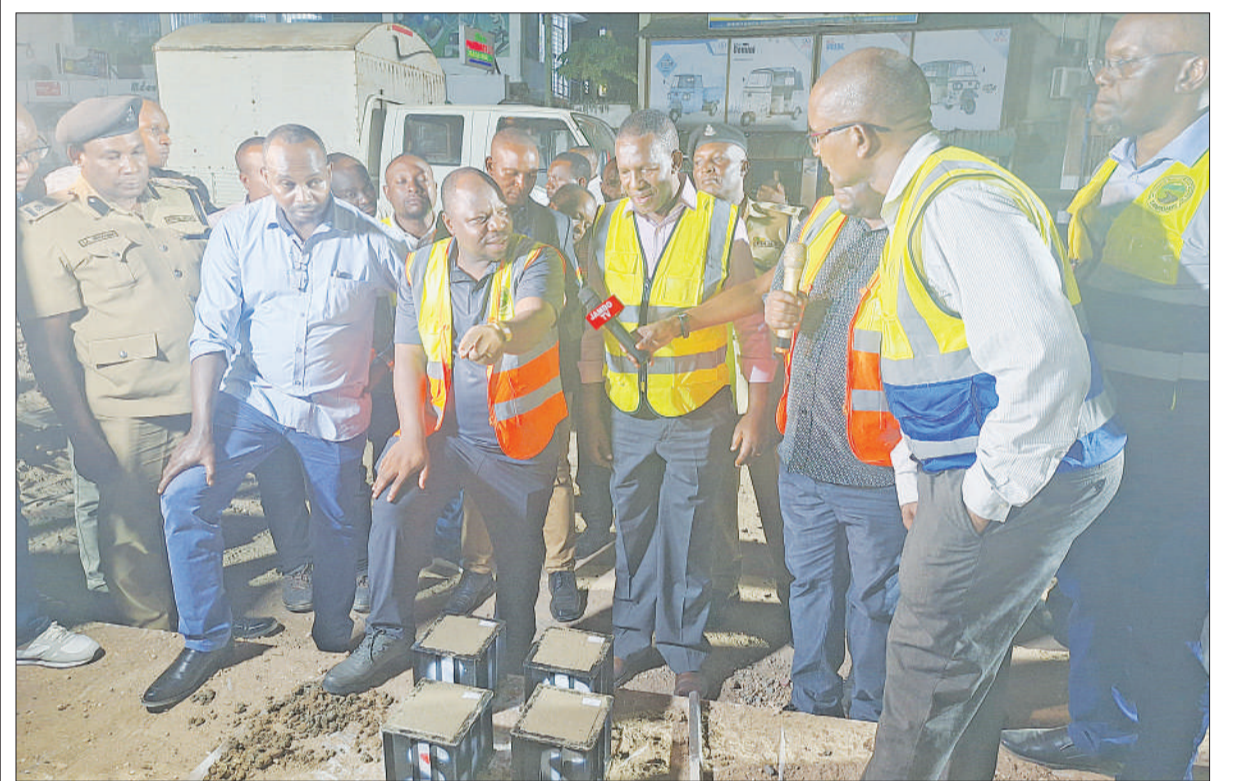
Dar es Salaam Regional Commissioner Albert Chalamila, speaks to Tanzania Roads Agency officials last night on the construction of the Bus Rapid Transit (BRT III) project during his night tour of various areas of the city to inspect development projects. Photo: Correspondent Joseph Mwendapole
