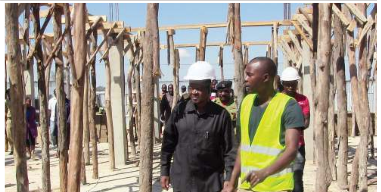
Tanzania Building Agency official Haruna Kalunga (R) briefs Rukwa regional commissioner Joachim Wangabo, who was on an inspection visit to the Kalambo district director's office yesterday. Photo: Guardian Correspondent
