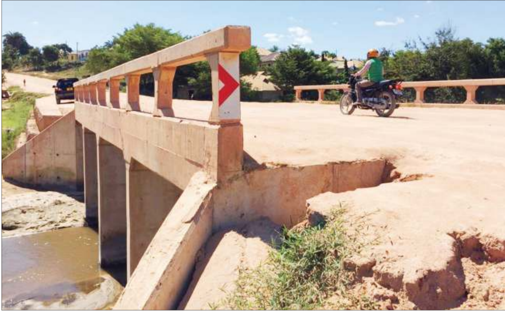
Kivule Bridge, a crucial link for Dar es Salaam's Kitunda and Kivule wards, is in need of urgent repair following damage caused by the recent heavy rains. This scene was captured yesterday. Photo: Correspondent Maulid Kambaya
