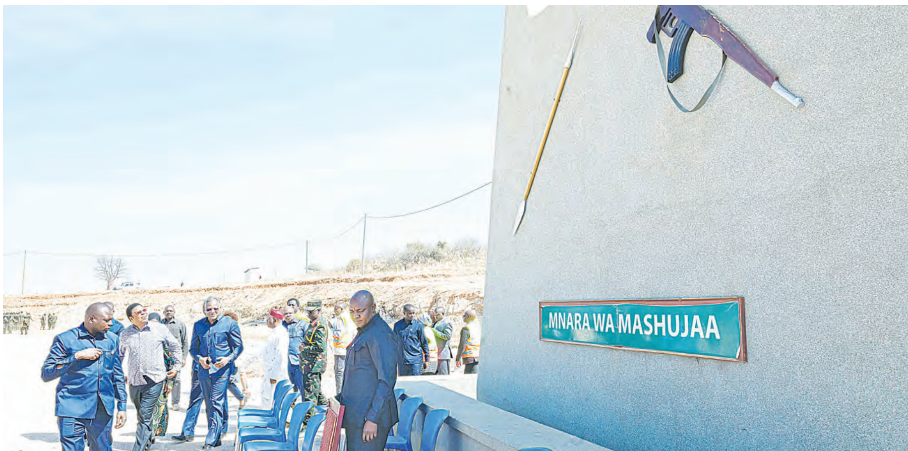
Prime Minister Kassim Majaliwa assesses progress in the construction of Heroes' Monument at Dodoma city's Mtumba Government Town yesterday, as preparations for this year's edition of celebrations to mark Heroes' Day (July 25) scheduled to take place in Dodoma Region at the national level continued. Photo: PMO
