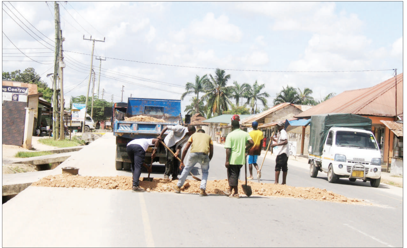
A team deployed by the Tanzania Rural and Urban Roads Agency moves to install speed humps at a Kitunda suburb section of a road in Ilala District, Dar es Salaam, yesterday. Photo: Correspondent Jumanne Juma
