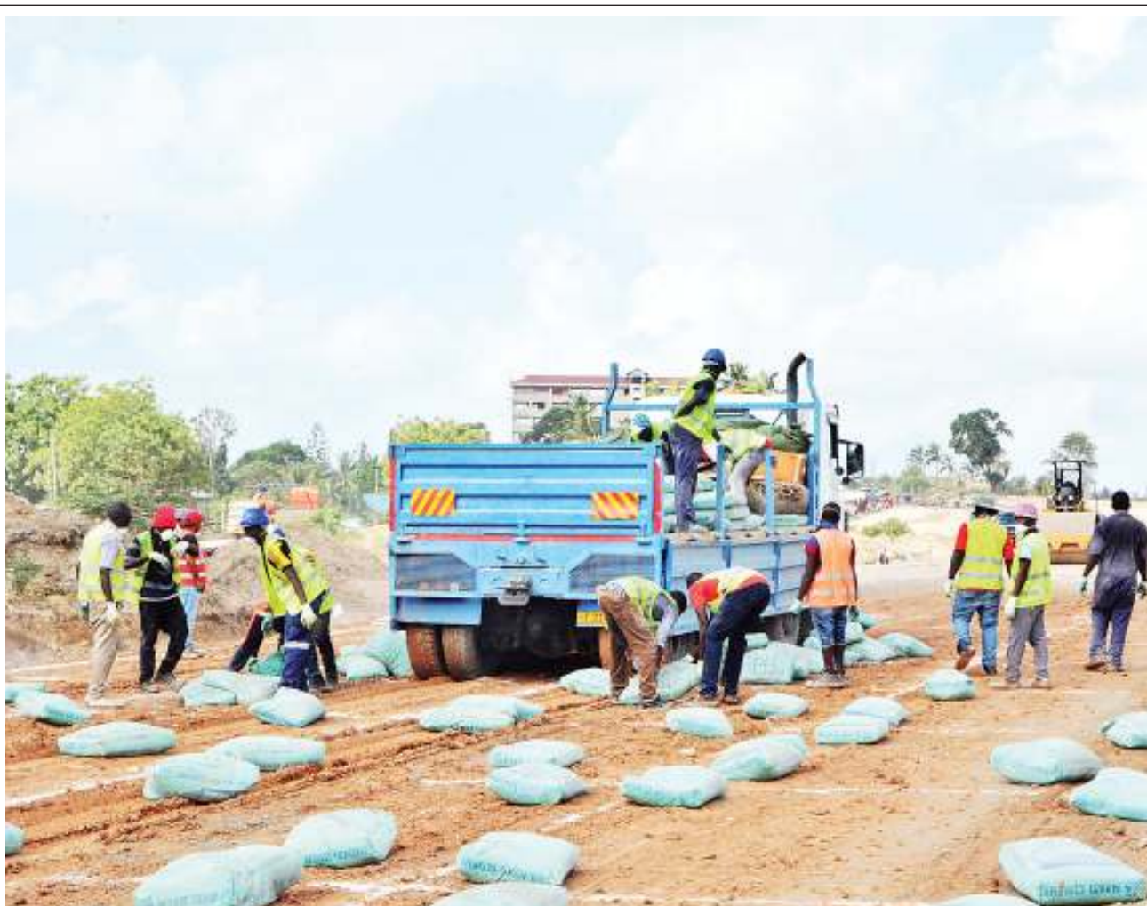
Preparations for major expansion of a section of the Kimara- Kibaha stretch of Morogoro Road to a six-lane structure in progress, as captured yesterday. Photo: Correspondent Miraji Msala
