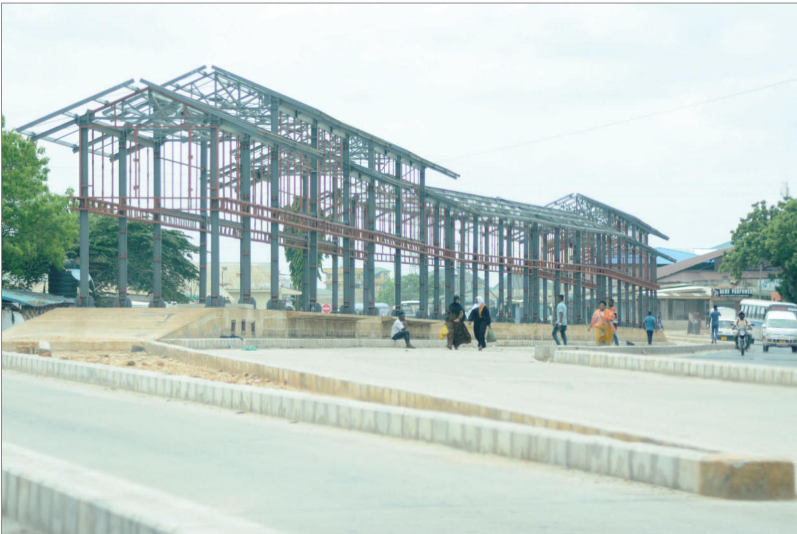
Aerial picture of the Dar es Salaam Rapid Transport bus stand which is under construction along Kawawa Road at Magomeni - Mikumi yesterday. Photo: Correspondent Jumanne Juma
