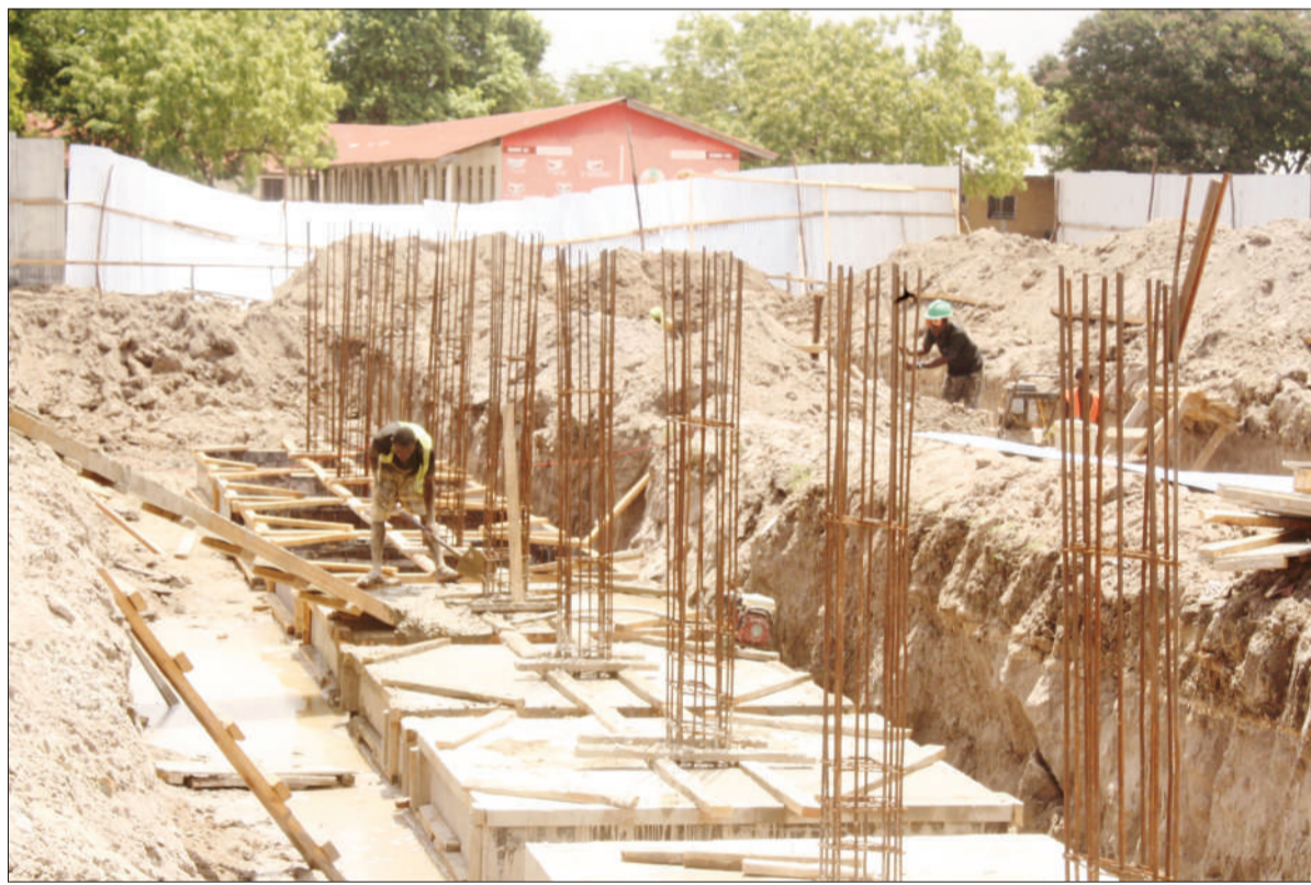
Pindoria Construction Ltd masons at the construction site of the second phase of Tabata Liwiti secondary school situated in Ilala district, Dar es Salaam region. About 20 class rooms are expected to be completed on time. Photo: Guardian Correspondent
