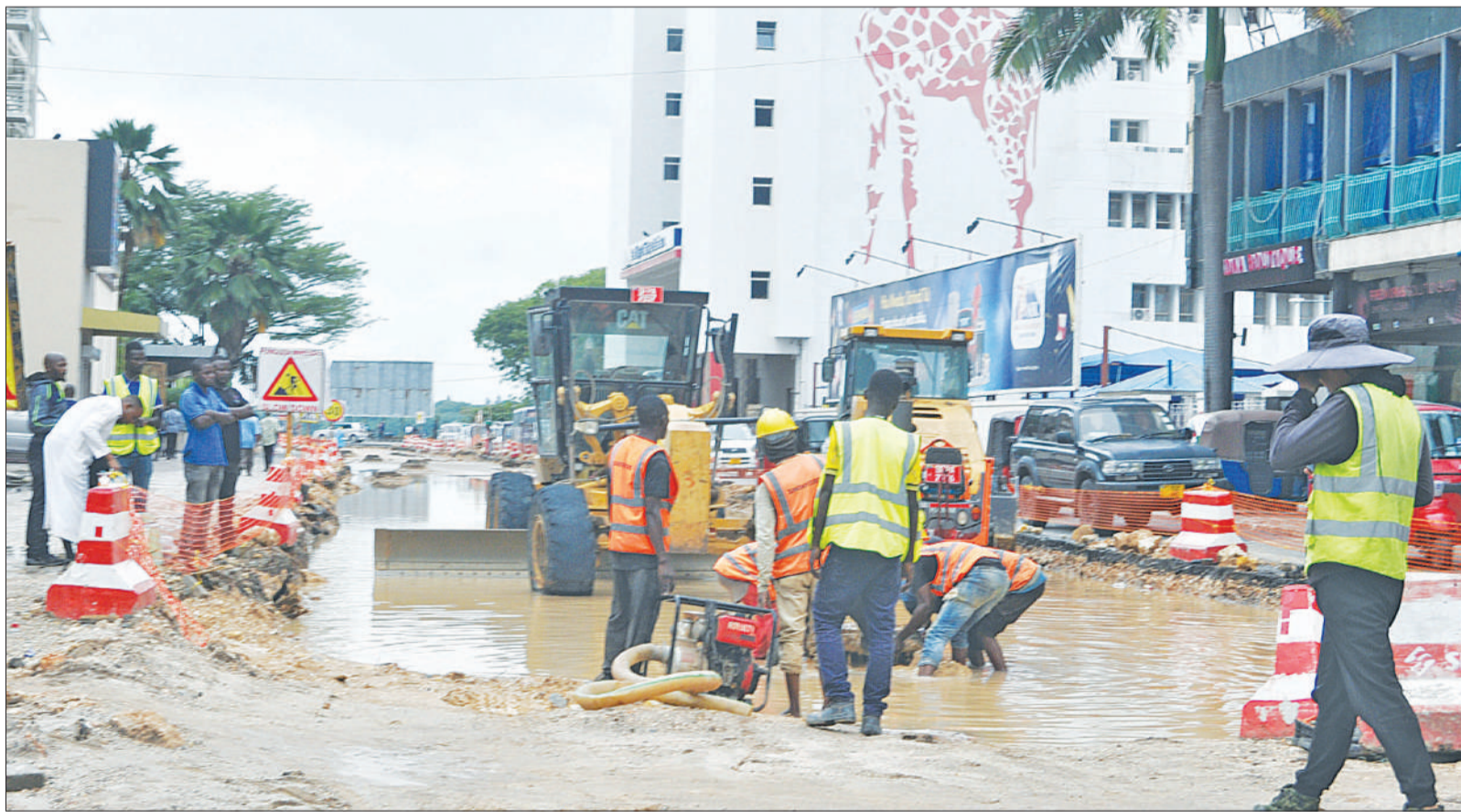
Implementation of Dar es Salaam's rapid transit bus infrastructure project in progress along downtown's Ohio Street yesterday, despite a downpour. Photo: John Badi
