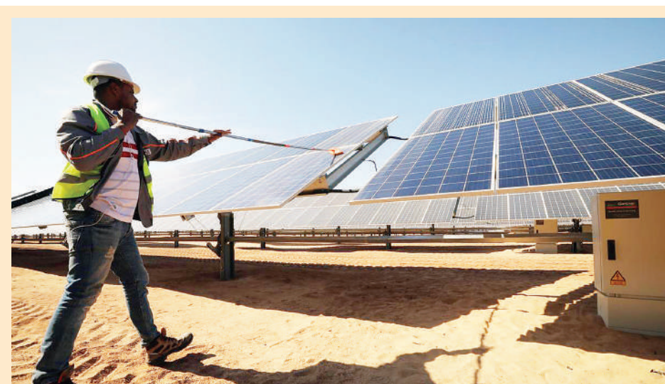
A man cleans solar panels at the Benban Solar Park in Aswan, Egypt.
