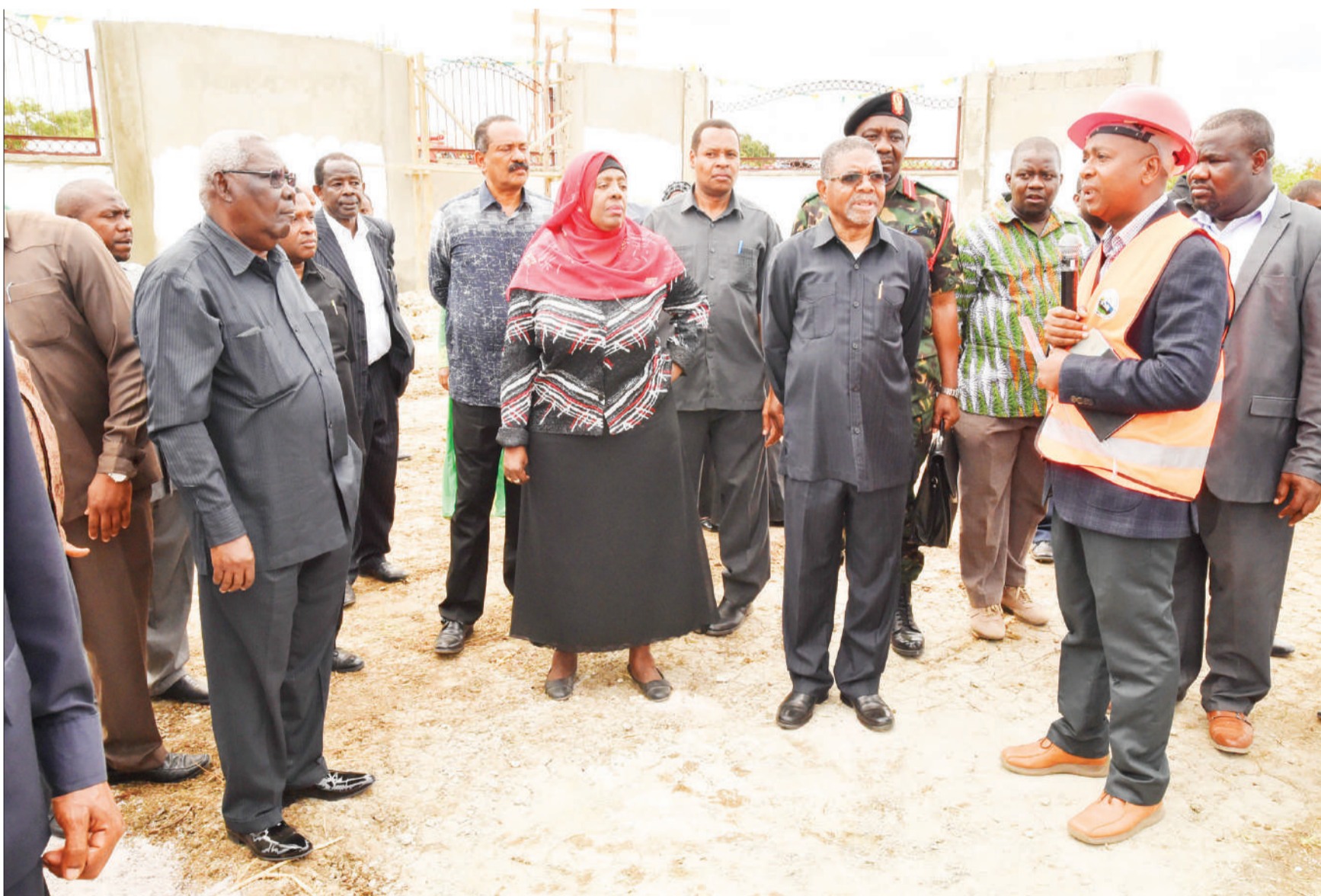
Zanzibar President Dr Ali Mohamed Shein visits a seaweed factory construction site at Mwani Chamanangwe in Wete on Pemba Island yesterday, accompanied by Zanzibar Second Vice President Seif Ali Iddi (L) and Zanzibar Industries and Trade minister Amina Salum Ali (C). Photo: Zanzibar State House
