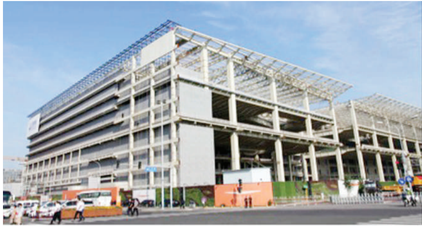
Photo taken on Sept. 5, 2020, shows the construction site of the second phase of the China National Convention Center project in Chaoyang district of Beijing. The main steel structure of the second phase of the China National Convention Center has been completed. (Photo: People's Daily Online)
