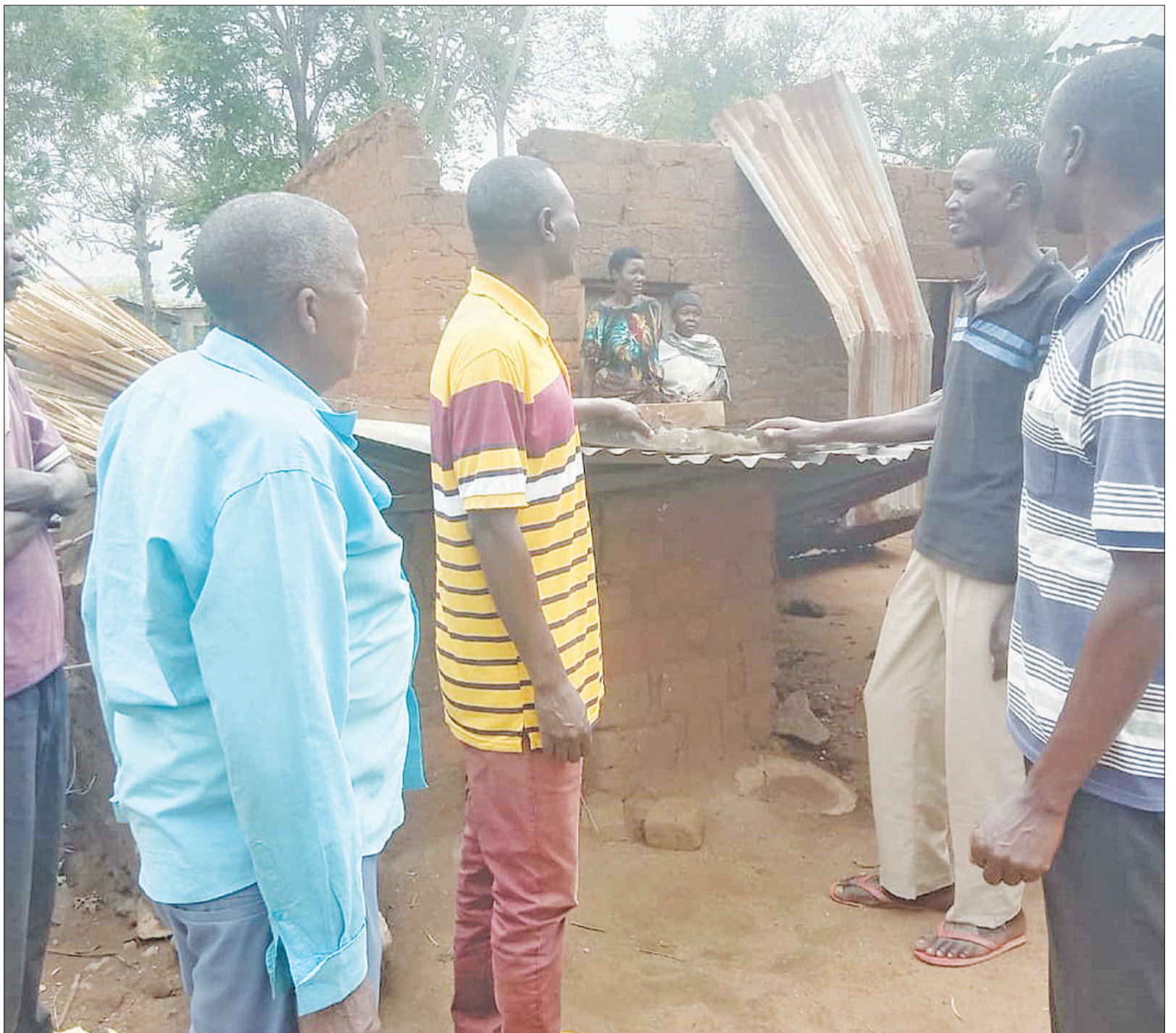
Residents of Suguti village in Musoma Rural constituency look on forlornly at the weekend at one of the houses damaged by a downpour. Photo: Guardian Correspondent
