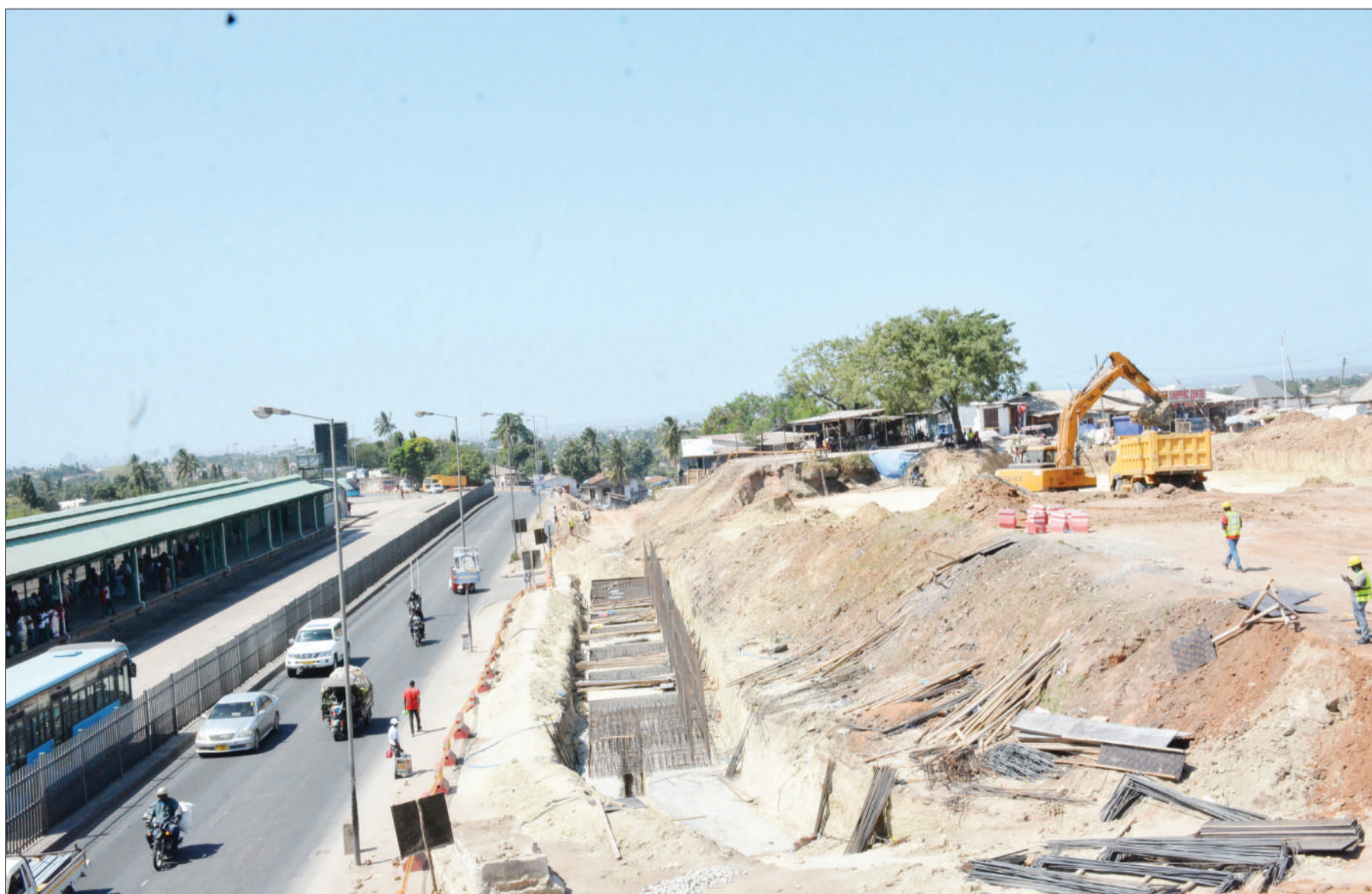
Kimara -Ubungu road widening project along the Morogoro Road highway in Dar es Salaam to ease traffic congestion going on well as captured by our correspondent yesterday. Photo: Miraji Msala
