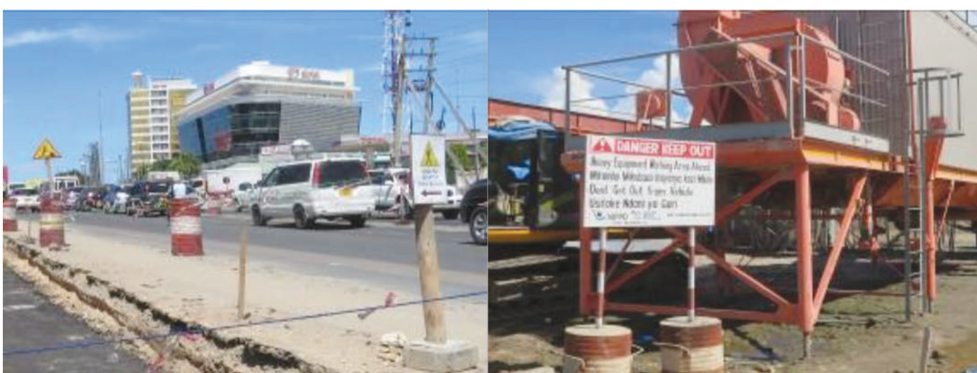
Safety sign boards written both in English and Swahili during project implementation
