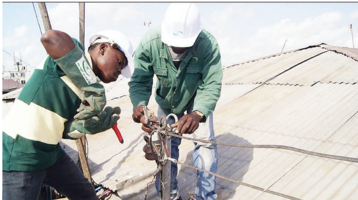
REA technicians installing power in one of the rural houses. (File photo)
