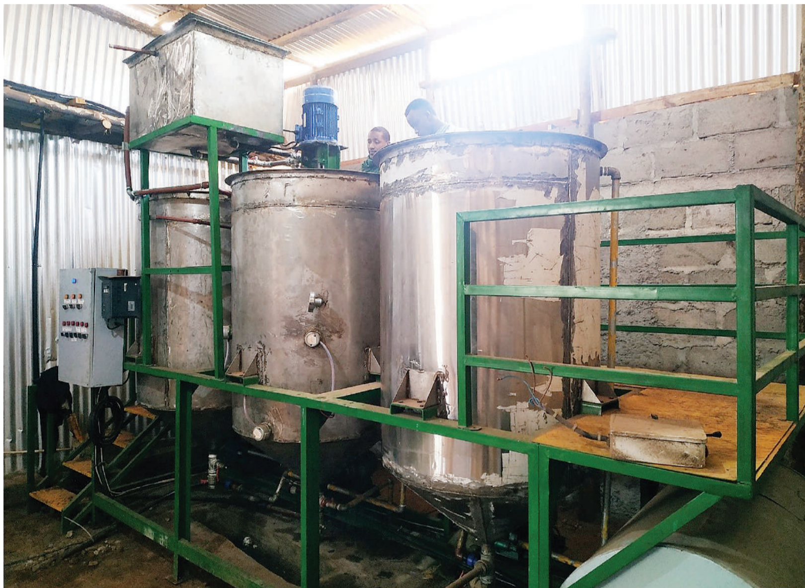
Engineers at TEMDO installing sunflower oil refining machine with 1000 litres capacity.
