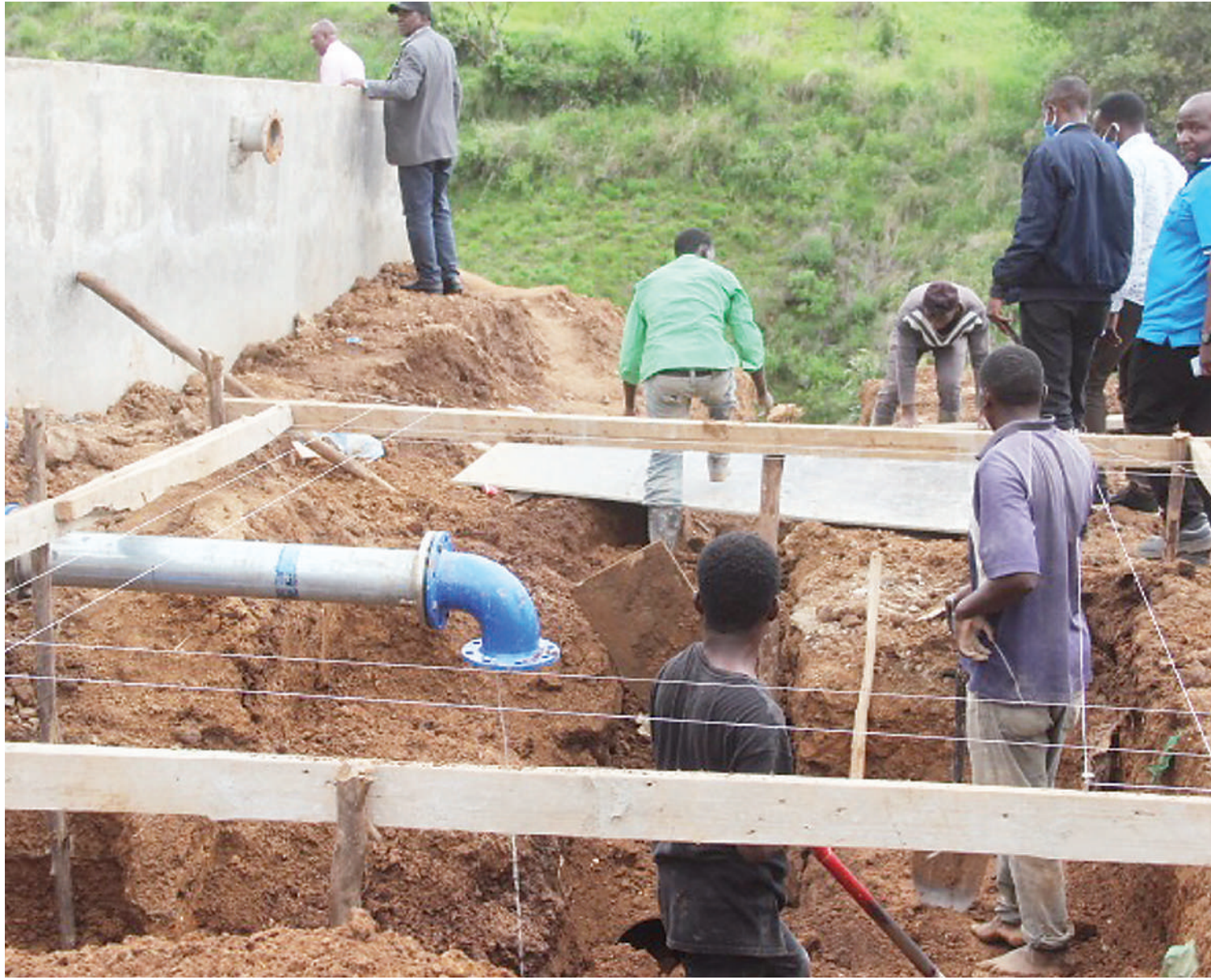
Implementation of Mbeya Urban Water Supply and Sanitation Authority's Mwashali-Isyesye water infrastructure project in progress, as witnessed yesterday. Sources said it is expected to be completed next week. Photo: Correspondent Nebart Msokwa
