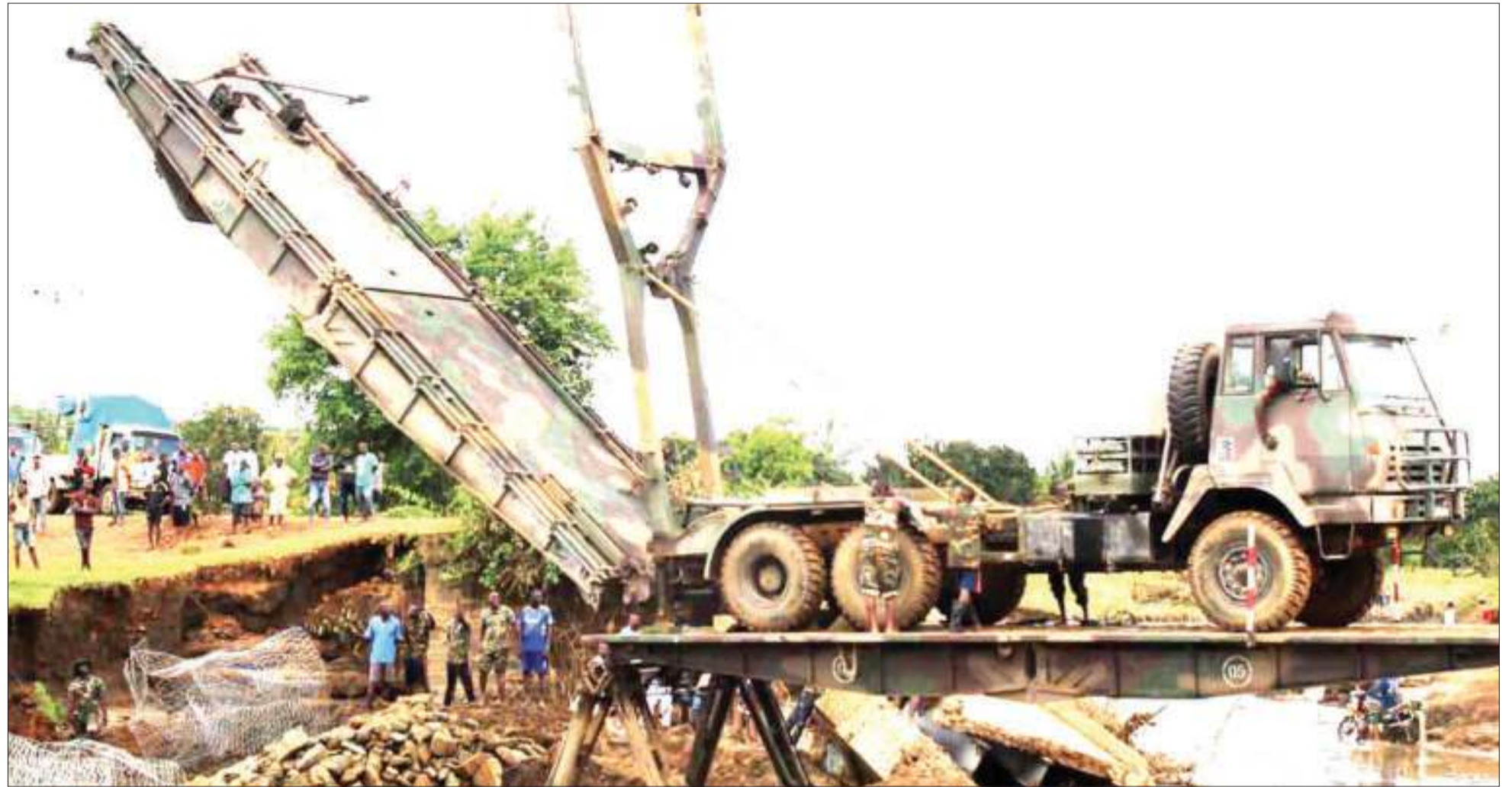
Members of the Tanzania People's Defence Forces move to install a temporary bridge across Nderema River in Handeni District, Tanga Region, as found at the weekend. The bridge previously there was recently swept away by floodwaters, which led to a serious disruption on transport to and from various parts of Tanzania and neighbouring countries. Photo: Correspondent Steven William
