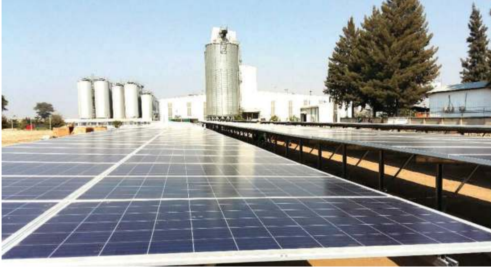
Solar power panels at TBL Mbeya plant. END
