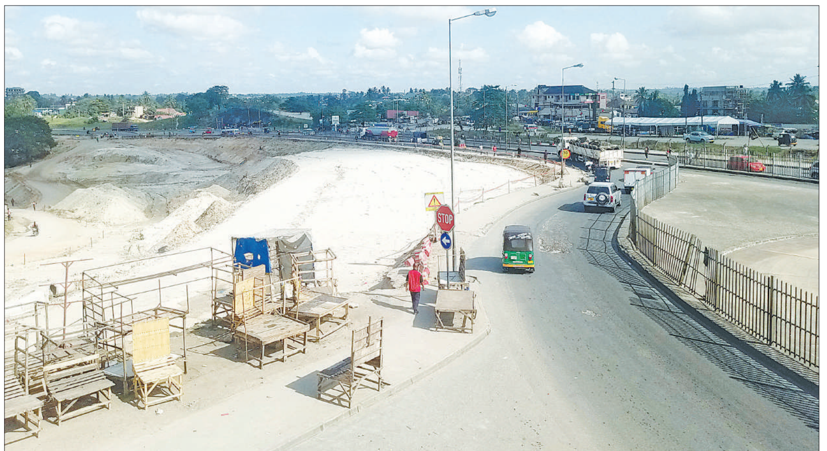
This is a view of Dar es Salaam's Kimara Mwisho valley, currently being filled with soil in readiness for the ongoing expansion of the Dar es Salaam-Kibaha stretch of Morogoro Road, as captured yesterday. Photo: Correspondent Sabato Kasika
