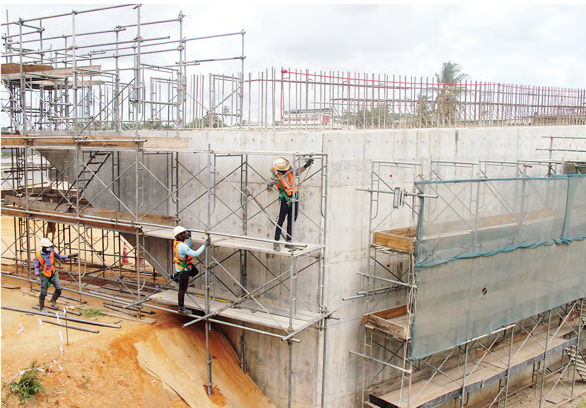
Implementation of the Dar es Salaam bus rapid transit (DART) project in progress earlier this week with the construction of a strategic bridge along the Mbagala-Gerezani stretch. Photo: Correspondent Jumanne Juma
