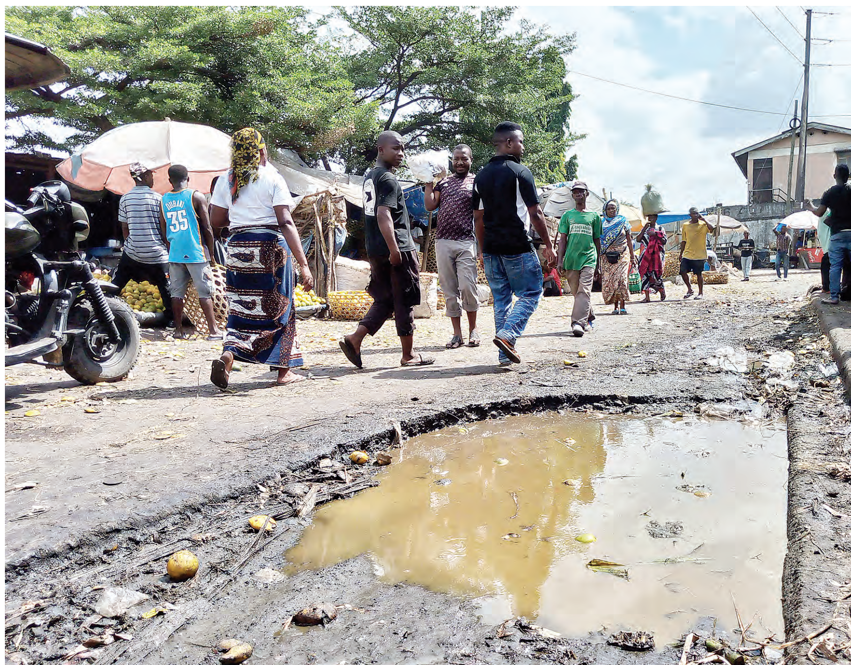
Motorists, pedestrians and small traders alike have for long found this badly damaged road at the backside of Dar es Salaam's popular mixed-goods market especially challenging, as Correspondent Sabato Kasika confirmed earlier this week.
