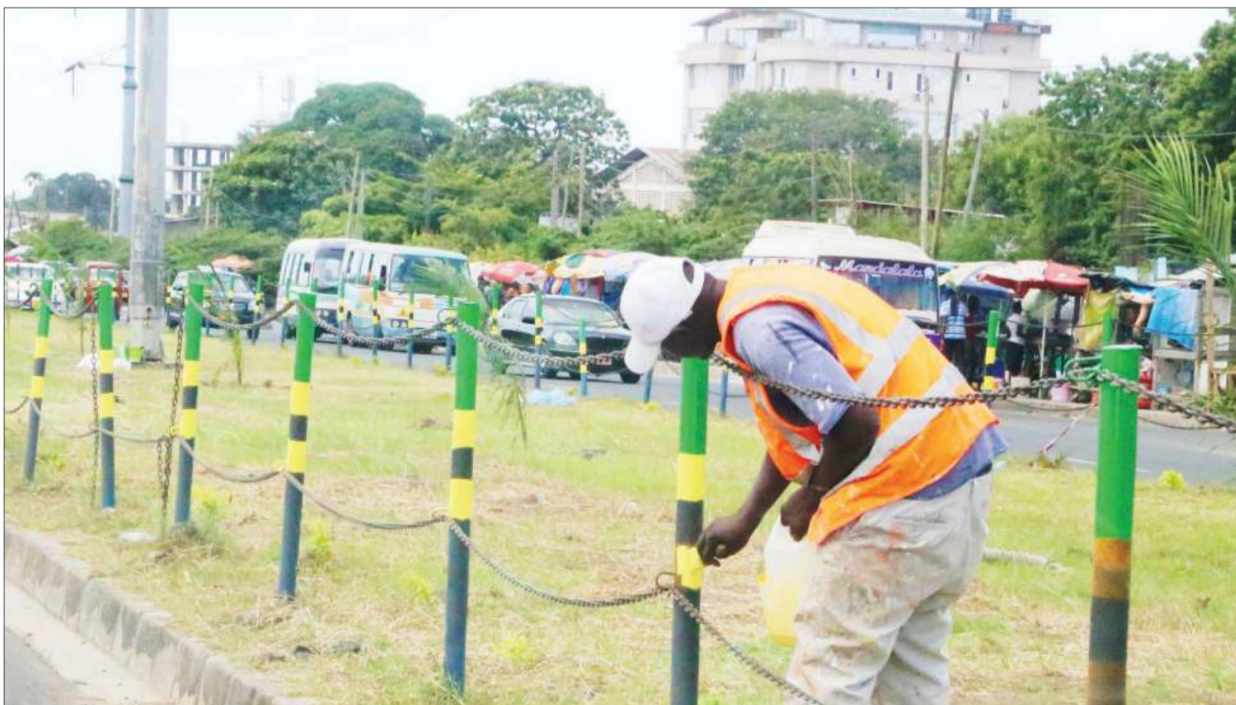
Kinondoni municipal painter at work along Sam Nujoma road in Dar es Salaam yesterday. Photo: Selemeni Mpochi
