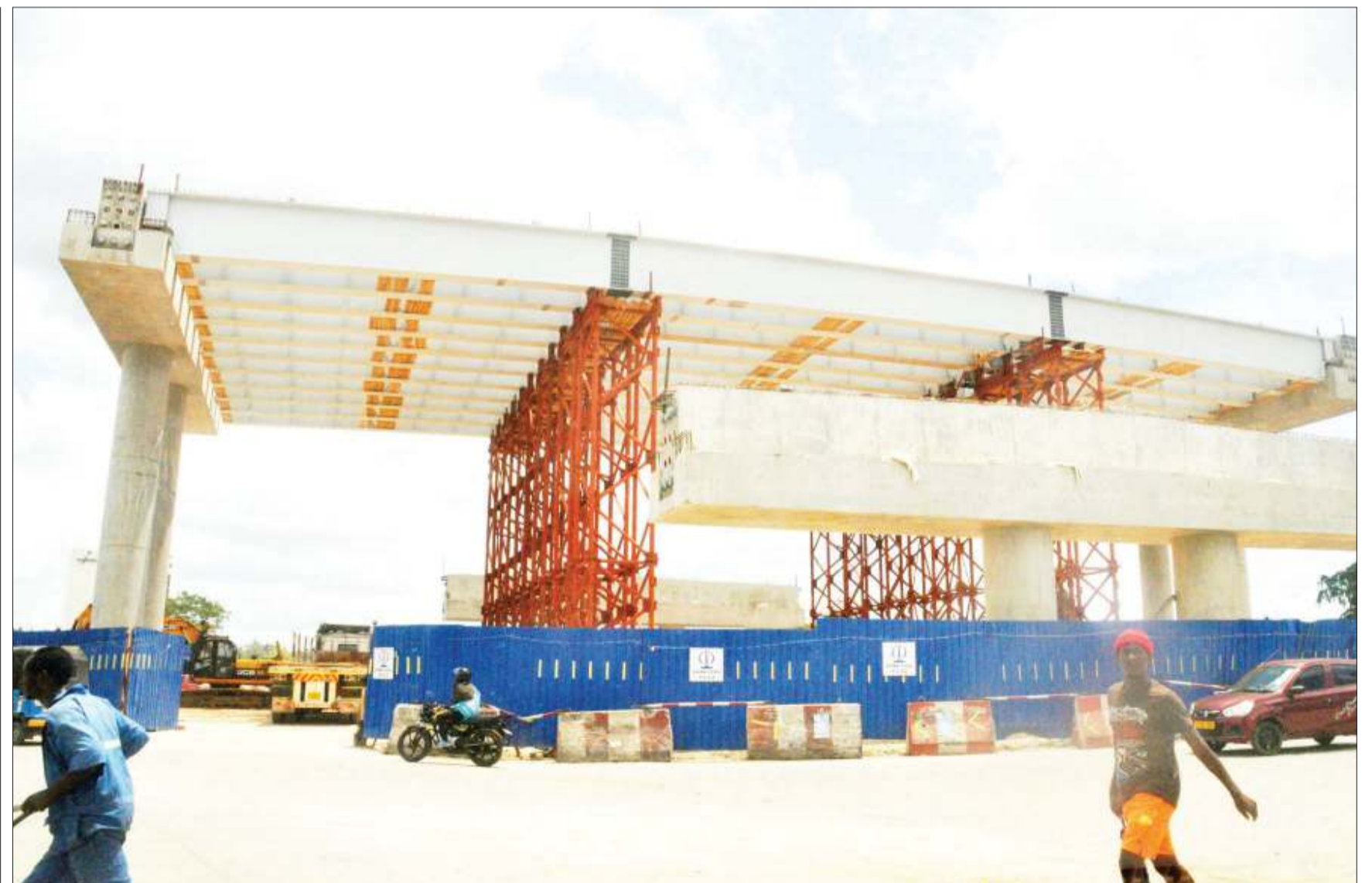
A view of the ongoing construction of Ubungo interchange at the roundabout of Morogoro Road/Mandela Express Highway as captured by our roving photographer in Dar es Salaam yesterday. The construction had reached 25 per cent and is expected to be completed by December 2020. Photo: John Badi
